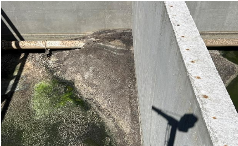
Basin #1 solids buildup
