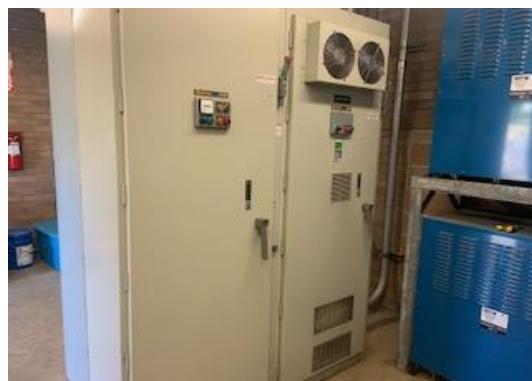
Fig 2: Variable Frequency Drive Panel
