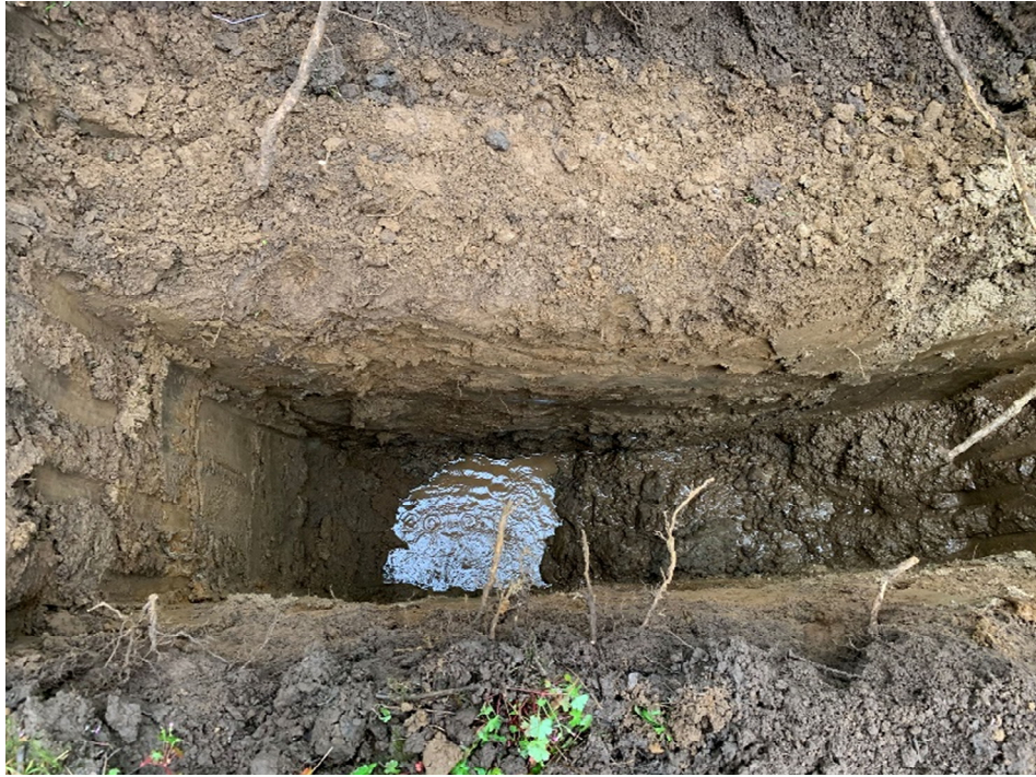
Photo 1. Seepage observed at TP-1.
