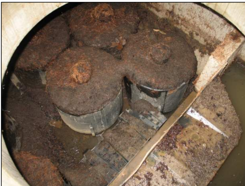
Media Cartridge Filter Vault with Accumulated Sediment
