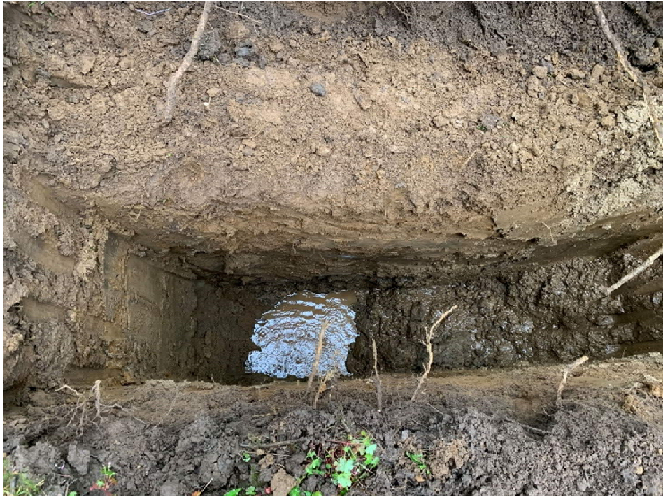
Photo 1. Seepage observed at TP-1.
