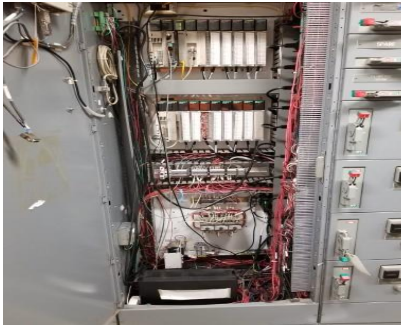
Figure 1: Existing PLC with wiring modifications over time
