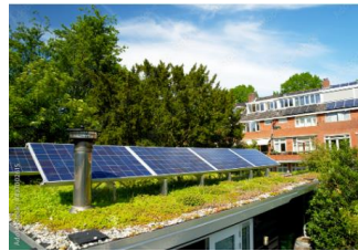
Solar panels on a green roof
