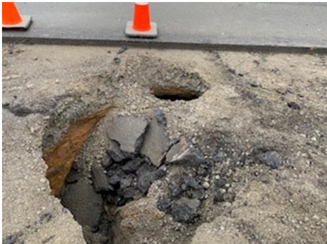
Figure 1. Sinkhole under Endicott St.
