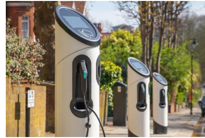
EV charging stations in curb zones (Source: © I-Wei Huang/ Adobe Stock)
