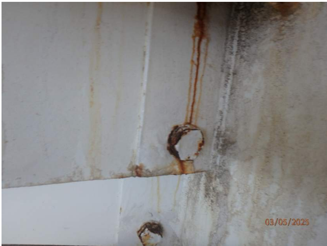
Figure 9: Heavy Corrosion of Bolt at Central Column
