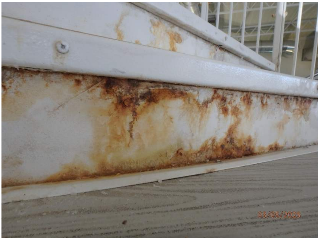
Figure 7: Heavy Corrosion with Scaling at Face of Riser
