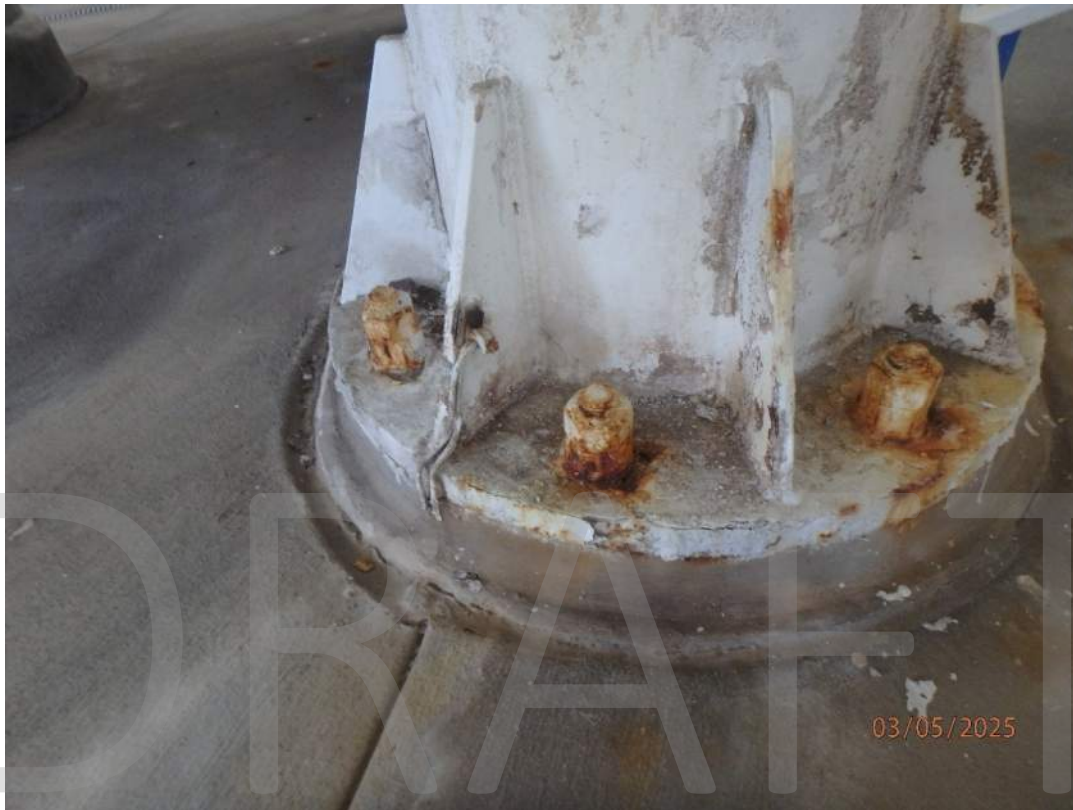
Figure 4: Typical Corrosion at Foundation Anchors
