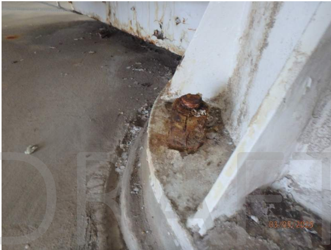
Figure 10: Heavy Corrosion at Foundation Anchors
