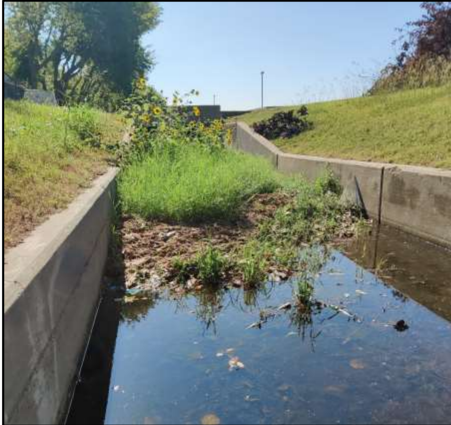
Clogged drainage along SW Murphy
