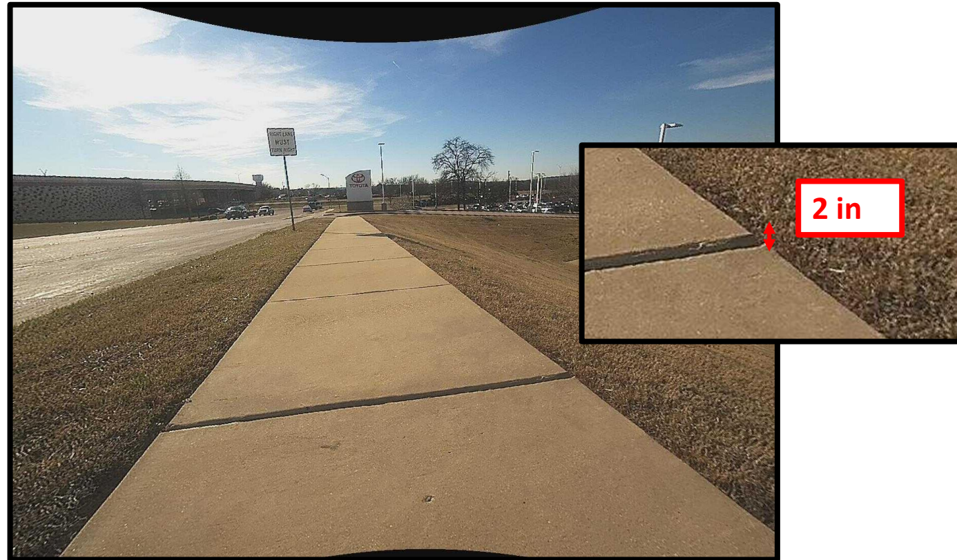
EXCESSIVE CROSS SLOPE AND TRIPPING HAZARD IN SIDEWALK PANELS (Sidewalk with Vertical Displacement greater than \frac{1}{4} in are non-compliant)
