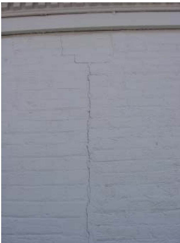
Fig 27: West elevation - Vertical crack at construction joint
