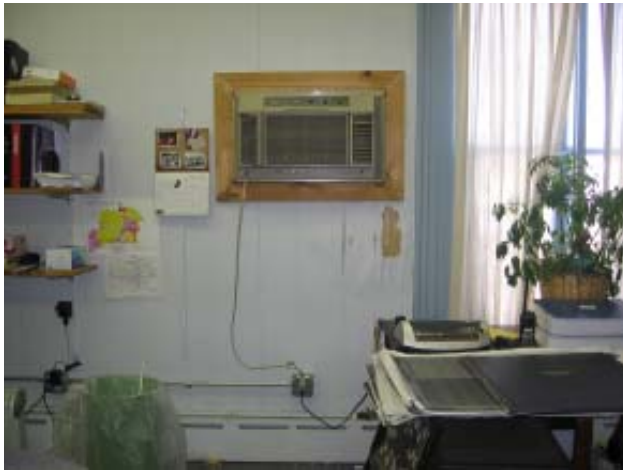
Fig 47: First Floor Level - Water damage below air conditioning unit in east exterior wall
