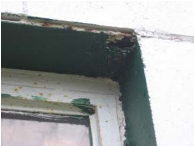
Fig 76: Garage- South elevation, rusting of steel lintel at man door
