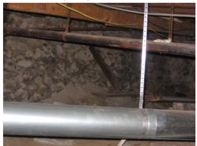
Fig 35: East Crawl Space - Wood bracing system along east exterior wall, excessive mortar dust pile
