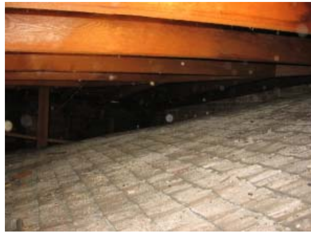
Fig 60: Attic and Roof Structures- Long span rafter splitting in west wing
