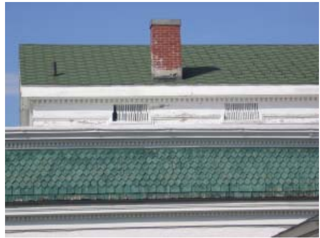
Fig 10: East elevation - Missing iron bar
