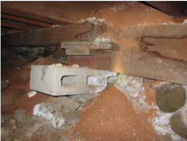
Fig 37: West Crawl Space - Excessive brick masonry dust at base of walls
