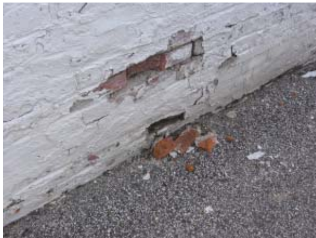
Fig 22: West elevation - Severely deteriorated brick
