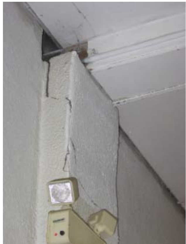
Fig 78: Garage - Masonry pier for roof beam bearing is cracked and rotating inward
