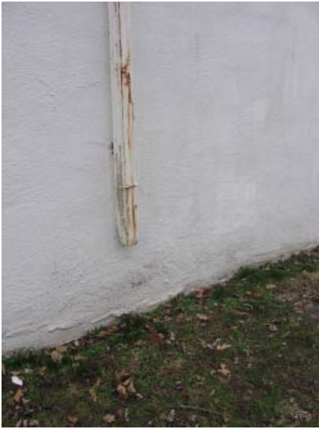
Fig 70: Garage- East elevation, downspout discharging against exterior wall of building
