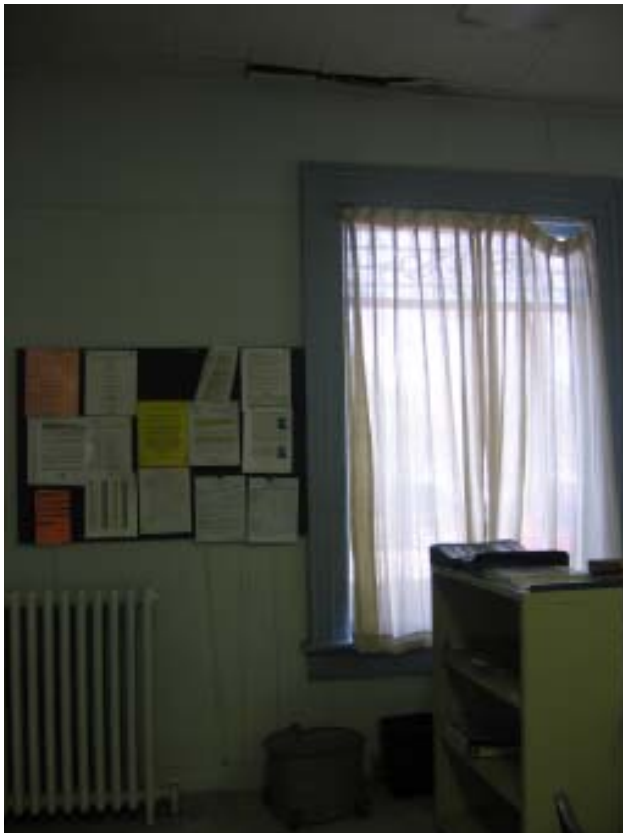
Fig 48: First Floor Level - Water damage at north wall of the east wing
