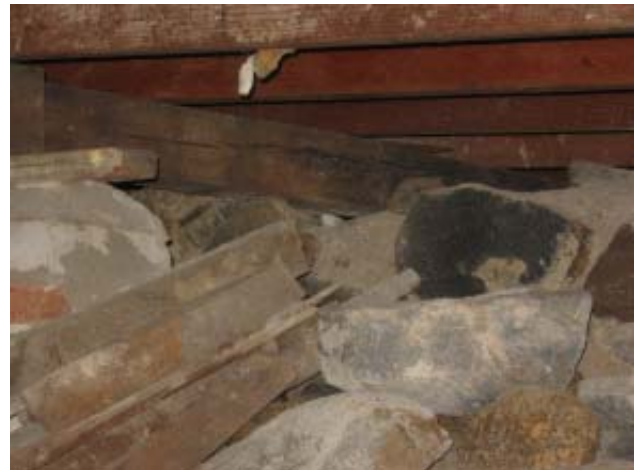
Fig 46: First Floor Structure - Deteriorated center beam in west wing
