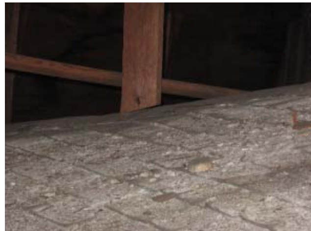
Fig 61: Attic and Roof Structures- Gap observed between bottom of stud supporting hip ridge and top of original hipped roof in west wing
