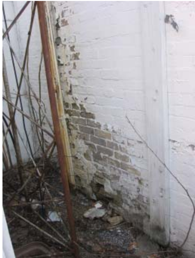
Fig 24: West elevation - Deterioration of brick at antenna enclosure
