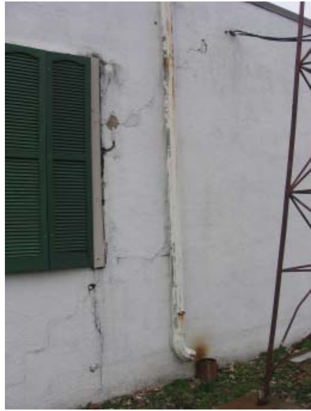
Fig 71: Garage- East elevation, downspout discharging against exterior wall and step cracking in masonry
