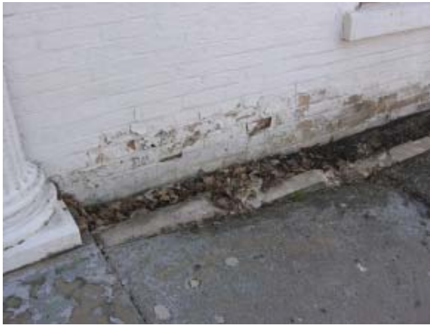
Fig 3: Deteriorating exterior brick north wall west wing
