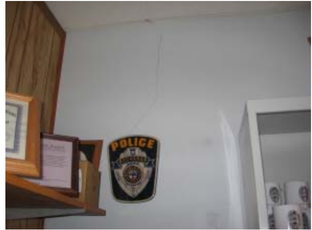
Fig 49: First Floor Level - Crack in west wall, north end of west wing
