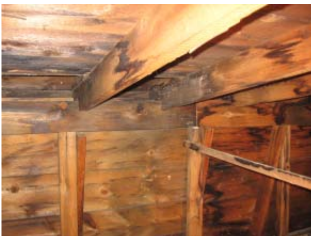
Fig 59: Attic and Roof Structures- Mansard roof construction details, note water staining in wood members in west wing
