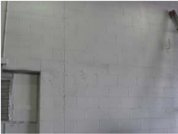
Fig 82: Garage - Vertical masonry crack in expansion joint on both interior and exterior surfaces of west wall
