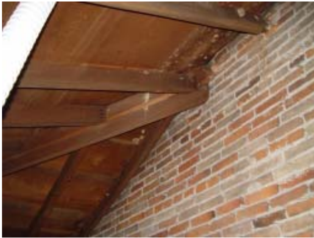
Fig 55: Attic and Roof Structures- Severely split hip ridge member at wall bearing, west wing
