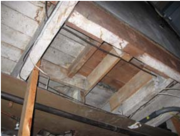
Fig 41: First Floor Structure - Floor infill at previous floor opening east of stair opening
