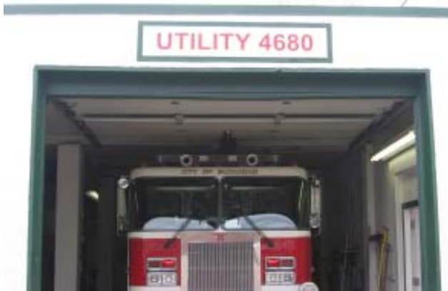
Fig 66: Garage- North elevation, visual sag in lintels
