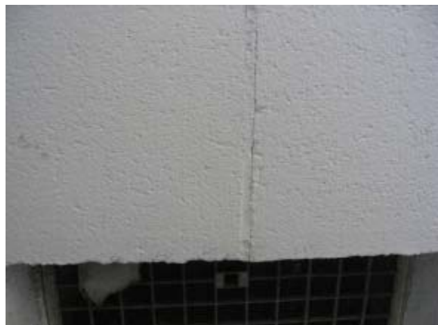
Fig 21: South elevation - Cracked cmu over vent
