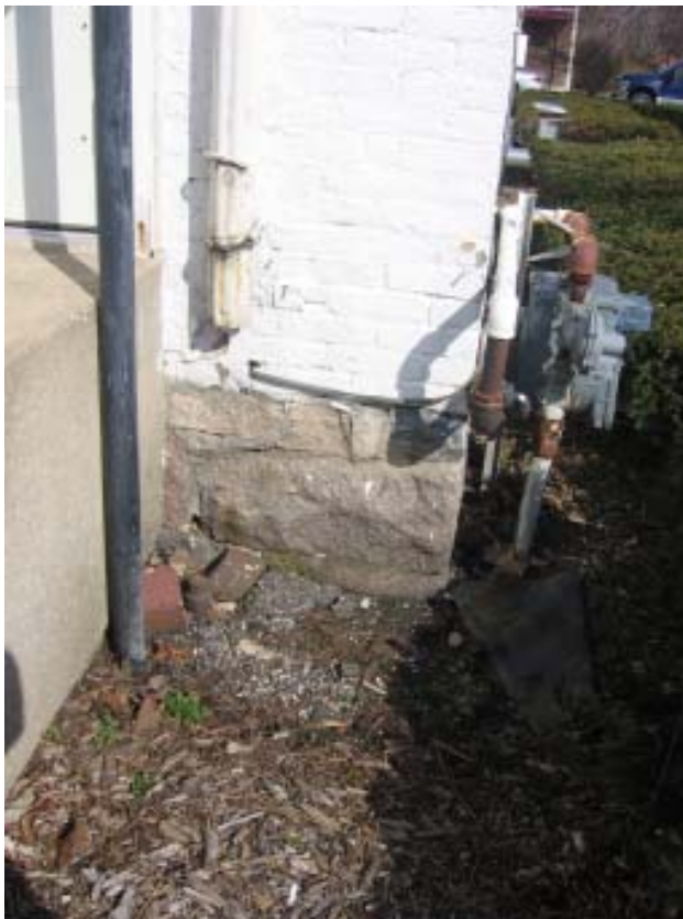
Fig 9: East elevation - Downspout discharging directly against foundation
