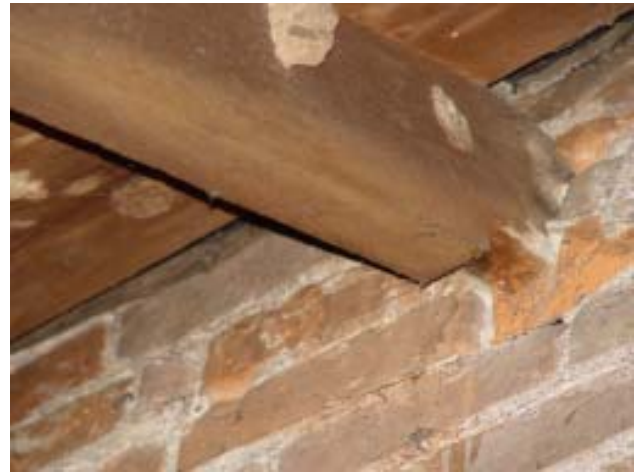
Fig 57: Attic and Roof Structures- Significant movement of rafters out of bearing pockets in west wing
