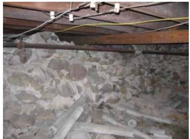
Fig 34: East Crawl Space - Stone masonry walls, excessive masonry dust presumed asbestos insulation
