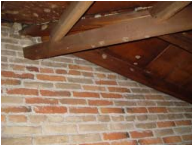
Fig 56: Attic and Roof Structures- Severely split hip ridge member at wall bearing, west wing
