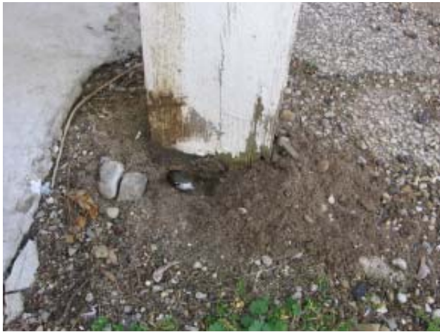
Fig 15: Carport column condition
