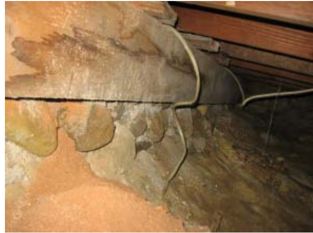
Fig 38: West Crawl Space - Excessive brick masonry dust at base of walls; loose stones in foundation wall
