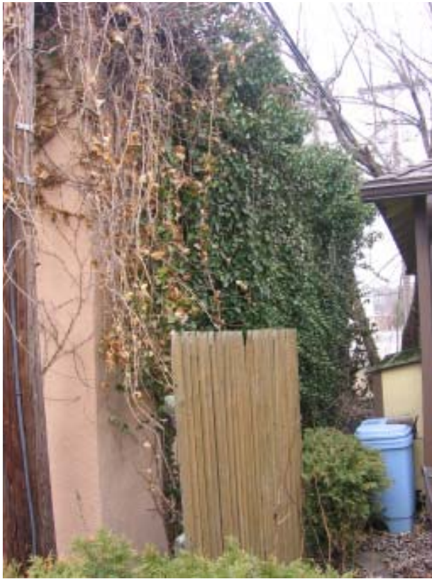
Fig 72: Garage- South elevation, heavy vegetation on wall prohibiting inspection of wall
