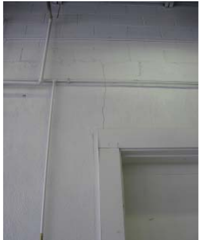
Fig 81: Garage - Vertical masonry crack in common wall between original and addition buildings; note stucco is discontinuous at new addition wall coursing
