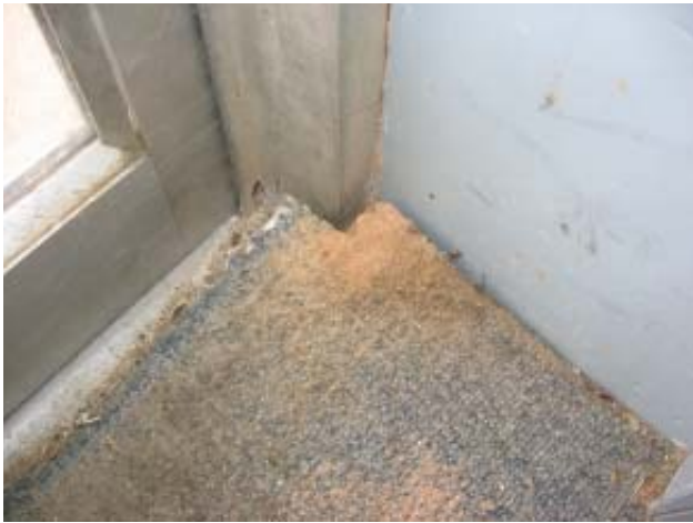
Fig 50: First Floor Level - Brick dust at man door in west wing
