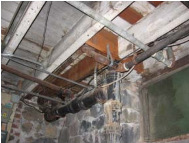
Fig 40: First Floor Structure - Floor infill at previous floor opening in southeastern corner
