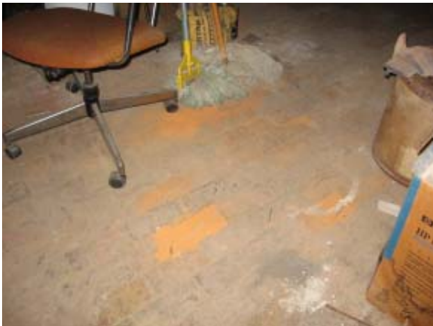
Fig 28: Basement - Deteriorated floor pavers
