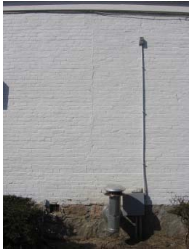
Fig 7: East elevation - Vertical cracked joint
