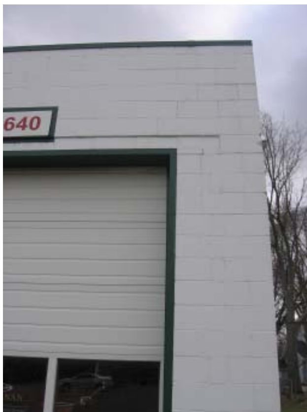
Fig 68: Garage- North elevation, step cracking at lintel bearing and western corner of wall
