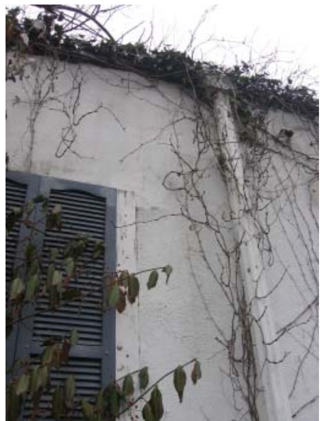
Fig 69: Garage- East elevation, heavy vegetation growth in gutter system
