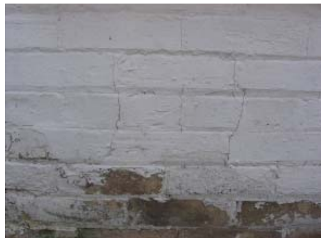
Fig 2: Cracking in exterior brick north wall west wing
