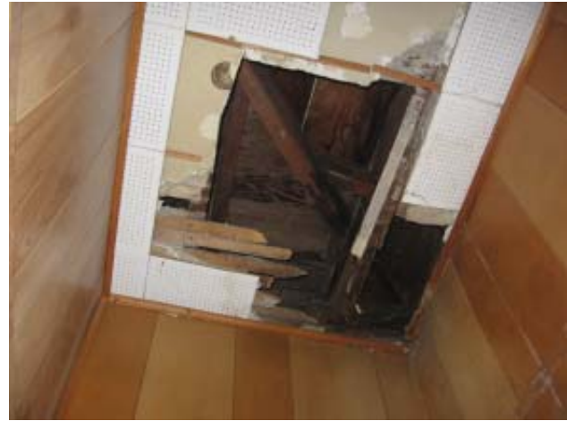
Fig 54: Attic and Roof Structures- Water staining in southeast corner of the east wing
