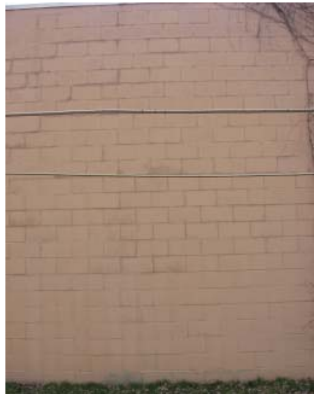
Fig 74: Garage- South elevation, south wall of addition cracking and moisture shown
