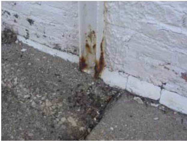
Fig 26: West elevation - Existing channel brace rusting
