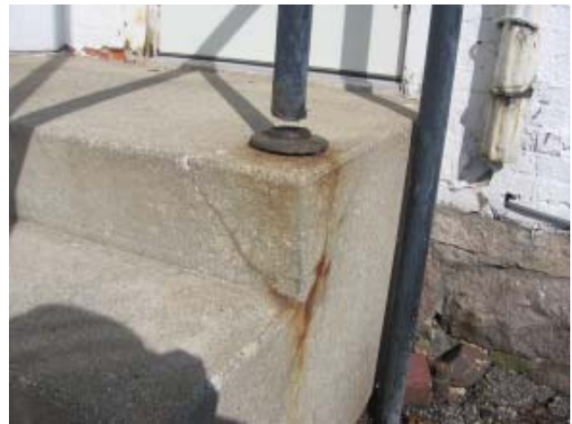
Fig 11: East elevation - Handrail support with no bearing
