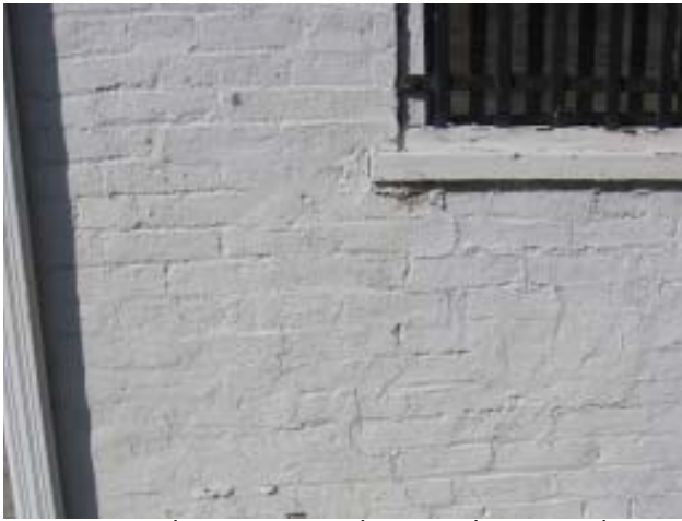
Fig 12: East elevation - Mainly vertical step crack
