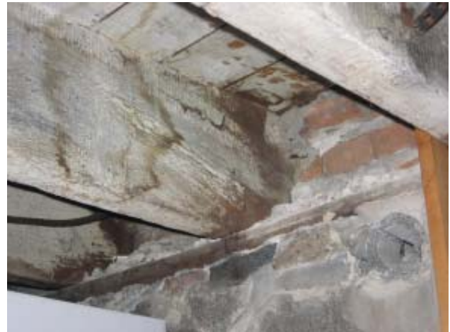
Fig 43: First Floor Structure - Cracked floor joist in northwest corner
