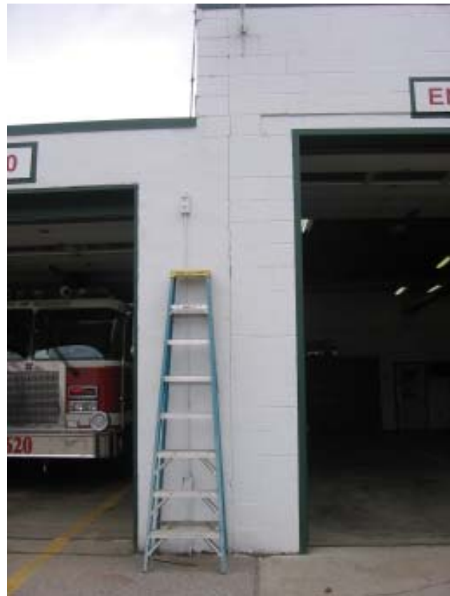
Fig 67: Garage- North elevation, vertical crack at joint between original and addition constructions
