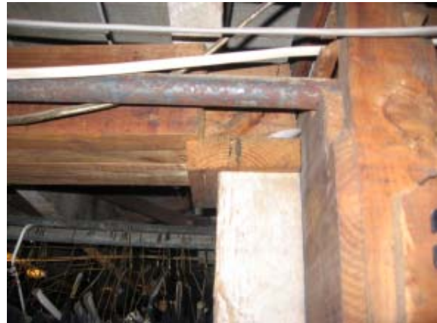
Fig 39: First Floor Structure - East beam line, south end, 3 of 4 plies have bearing on wood column
