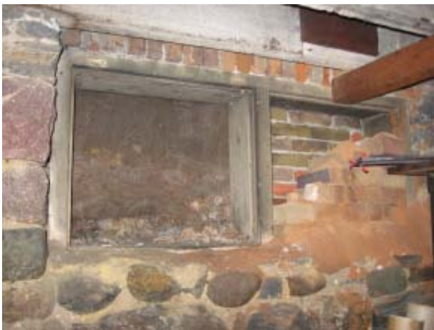
Fig 33: Basement - Window infill and deteriorating brick at north wall
