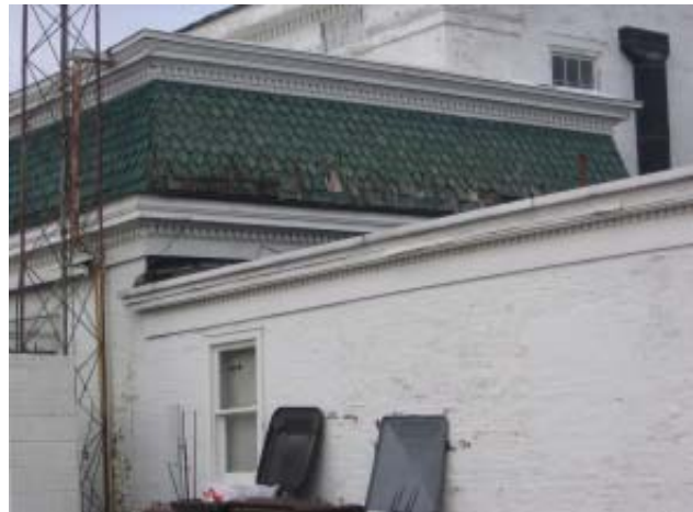
Fig 20: South elevation - Deteriorated shingles
