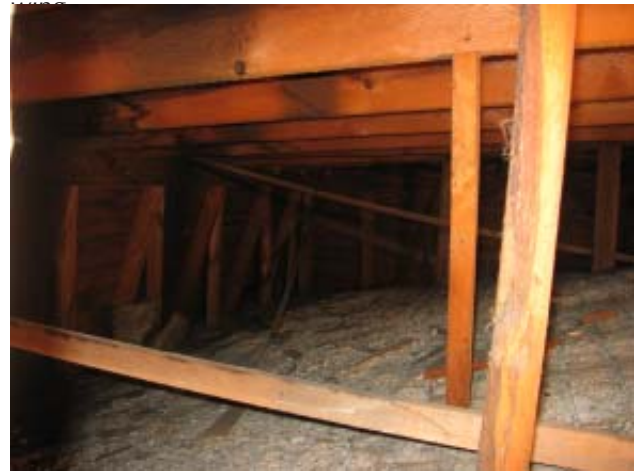
Fig 58: Attic and Roof Structures- Bracing of mansard roof construction of west wing
