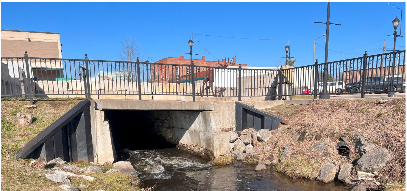
Figure 1: Image of failing culvert parallel to Days Avenue facing north (Buchanan, MI). Note: failure area inside culvert is approximately 10-20' into the culvert.
