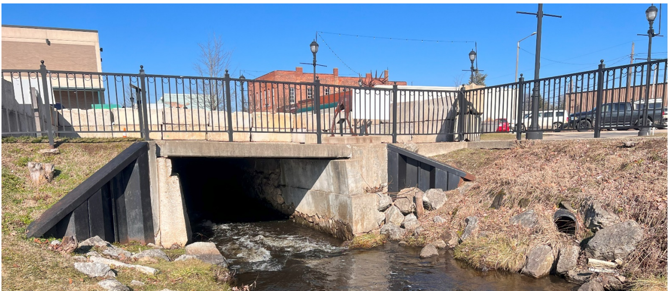
Figure 1: Image of failing culvert parallel to Days Avenue facing north (Buchanan, MI). Note: failure area inside culvert is approximately 10-20' into the culvert.
