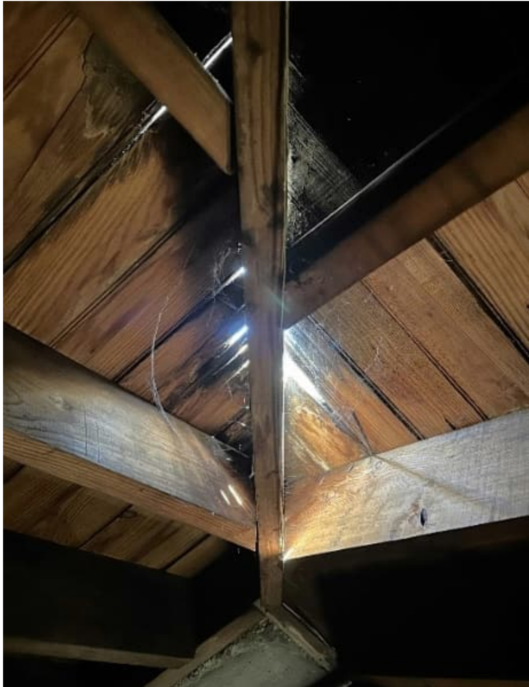
This photo shows deterioration of the house roof framing due to holes in the roof.
