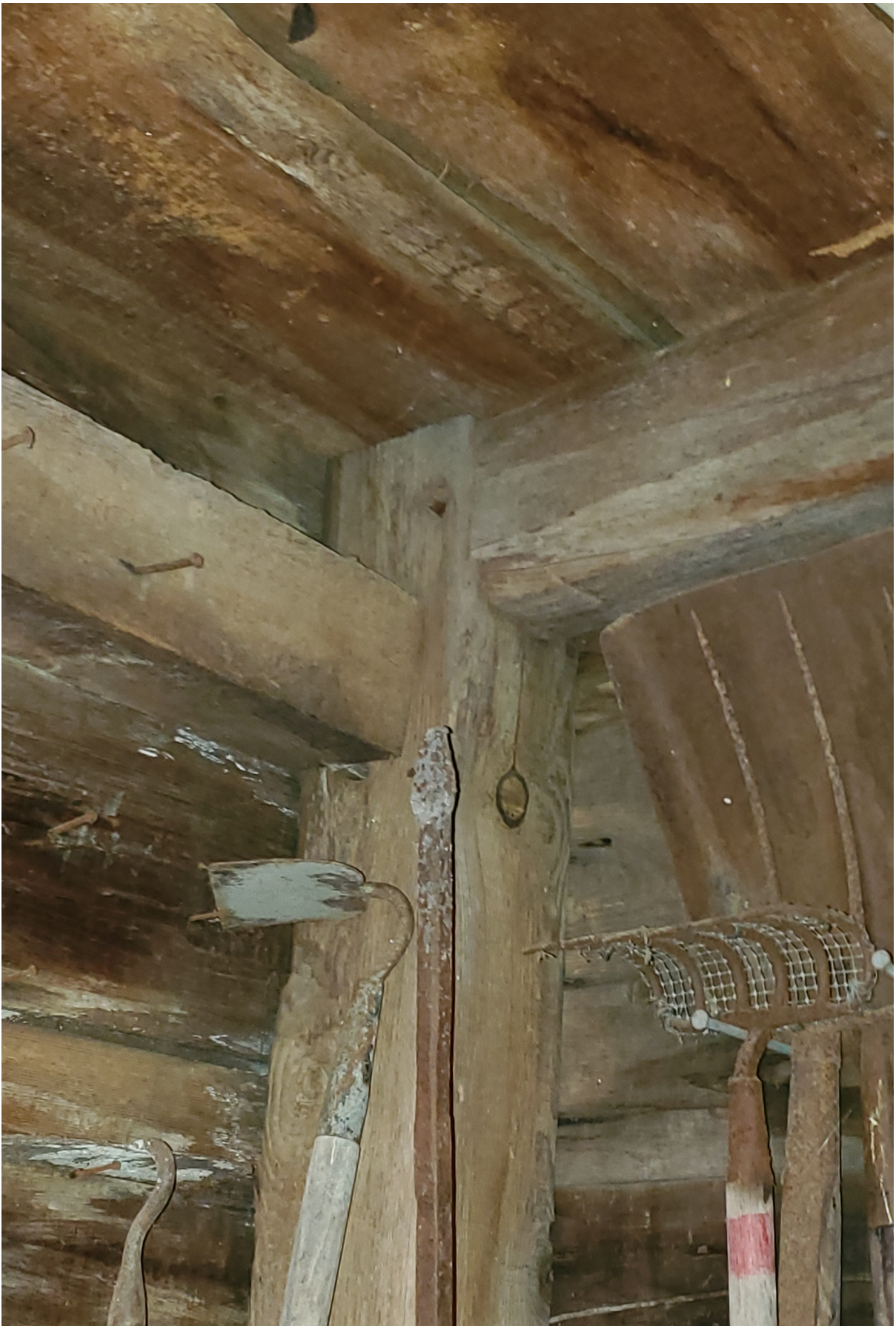
Figure 4: Corner post showing joinery and lack of corner bracing.
