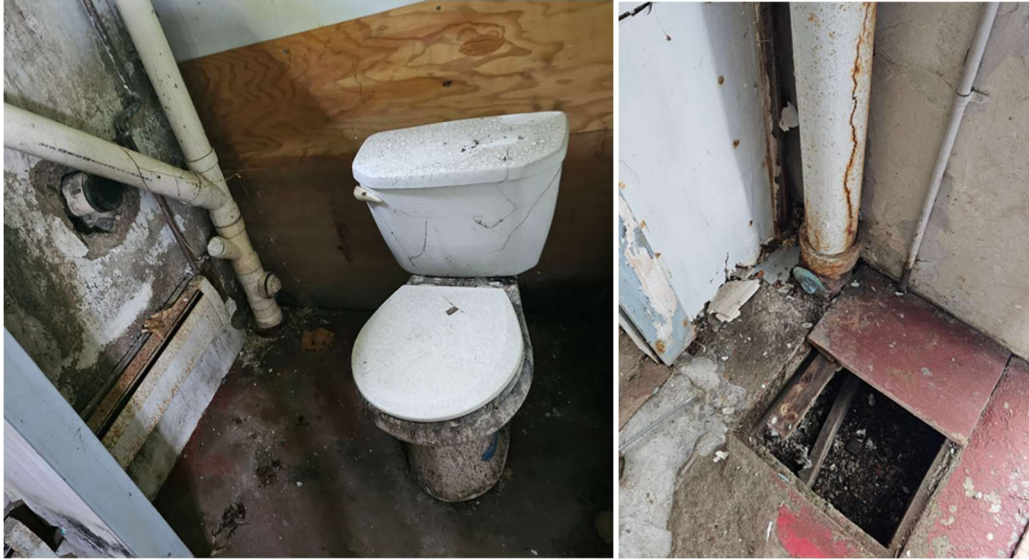
Image of basement waste lines.
