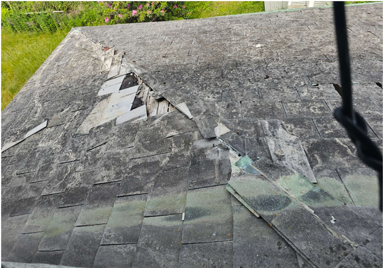
Image of garage roof, missing asbestos shingles reveal tar paper and plank sheathing.
