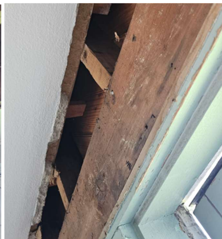
Image at first floor window header.
