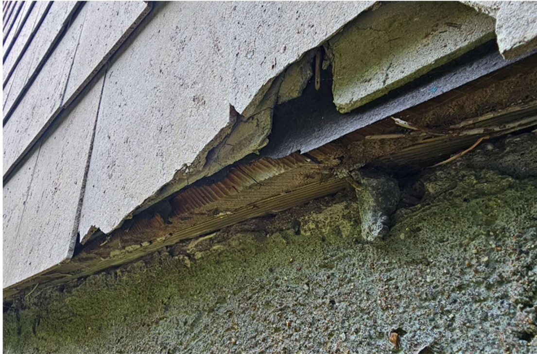
Image taken at exterior wall sill plate – note exposed wood framing is more prone to rot.
