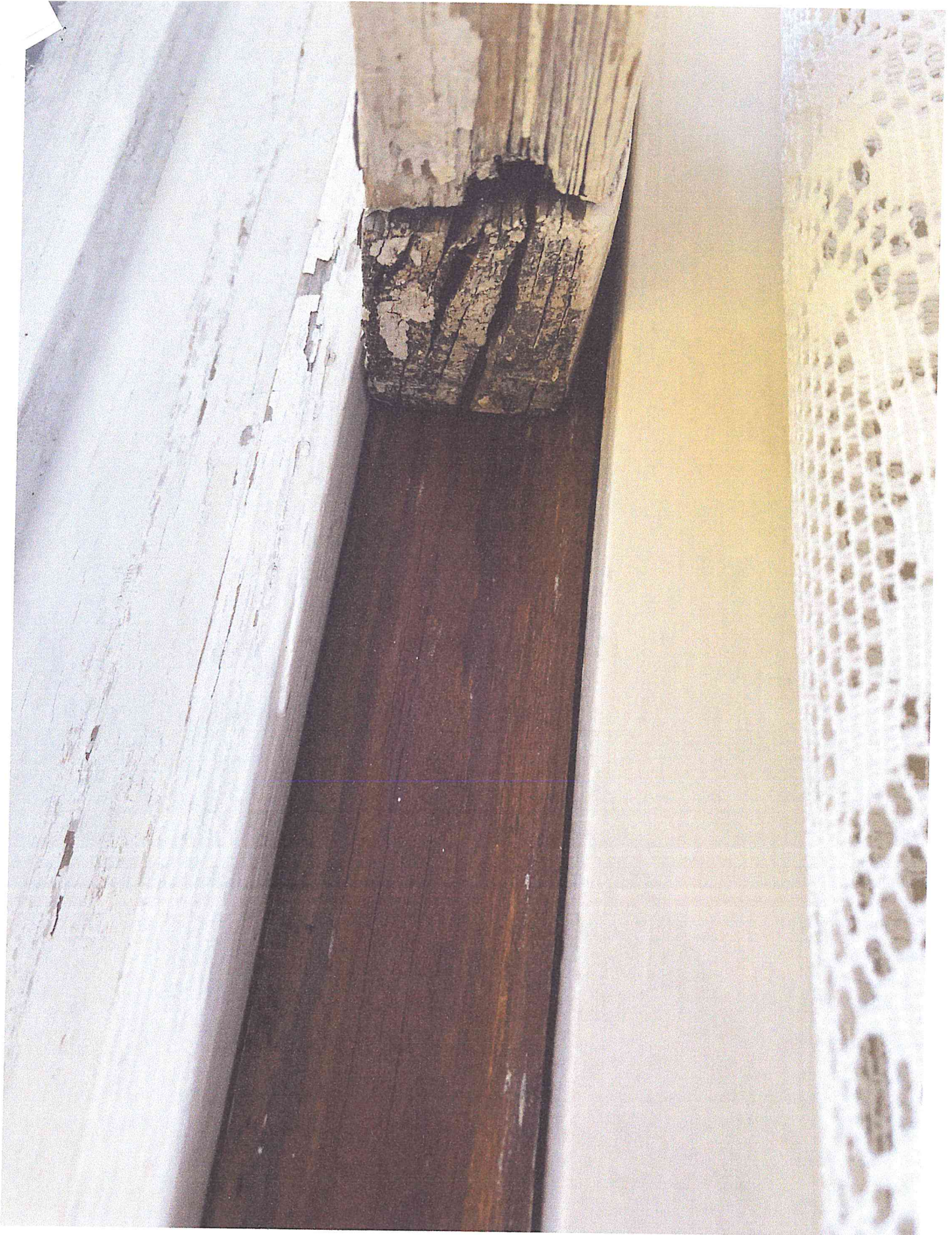
① DR LEFT OF 3 WINDOWS RIGHT SIDE OF LOWER SASH RAIL FROM BELOW: ROT
