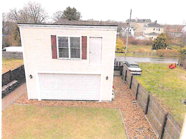
Current (No Access to only door except by ladder)
