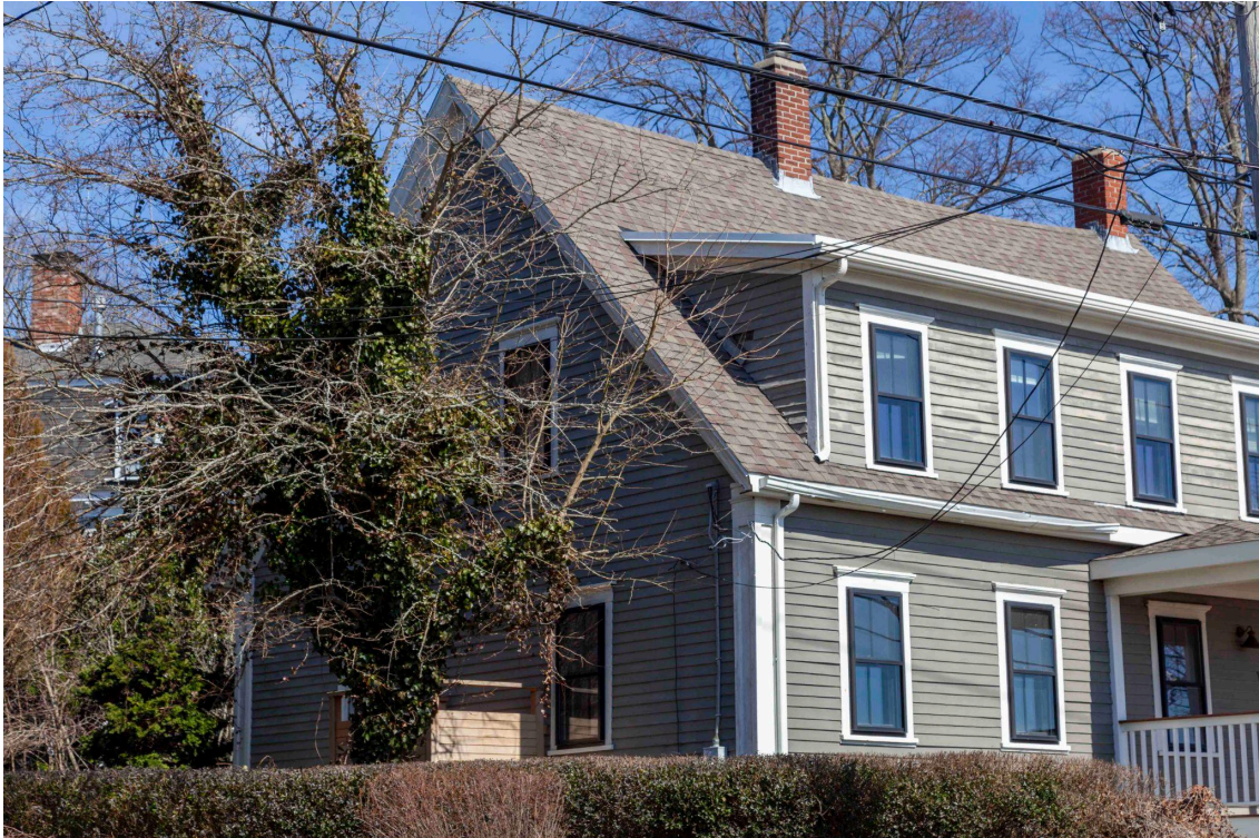
Photo 8 - Existing Roof Above Existing Dormer to Have New Porthole Windows
