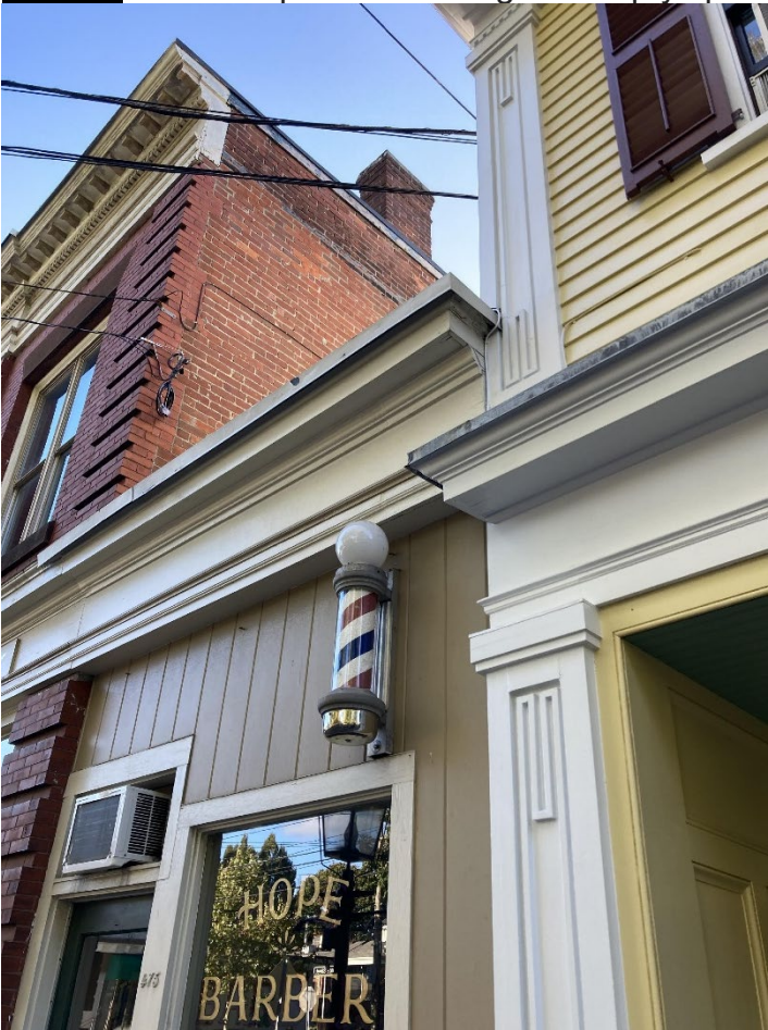
Photo 4 – Close up view showing the empty space above the Hope Barber Shop.
