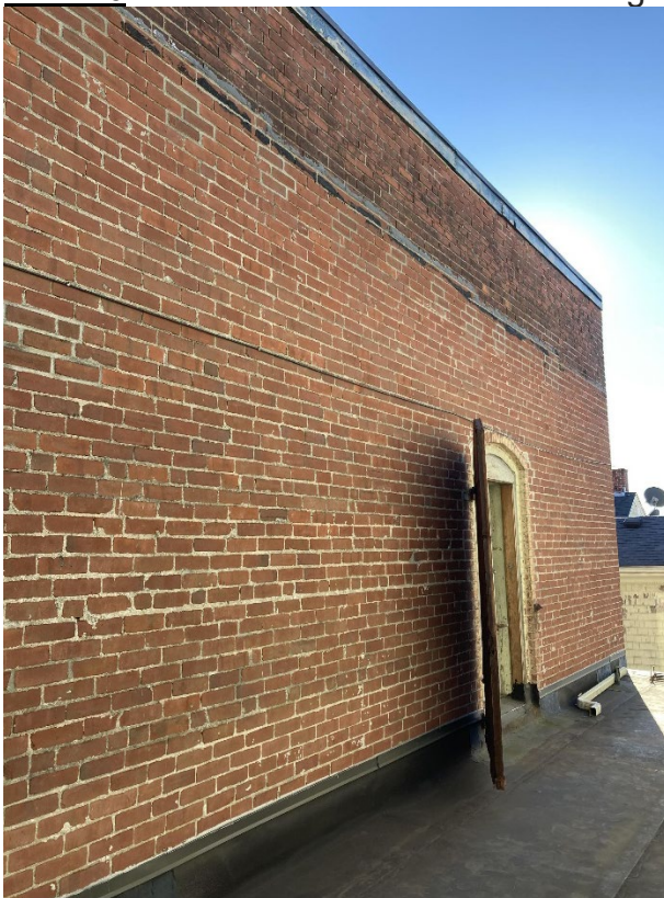
Photo 6 - Remnants on the brick showing location of non-surviving roofline.
