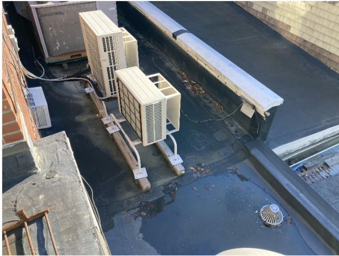
Photo 9 – Image showing rear lower roof over single story section of building where the current mechanical units are located.
