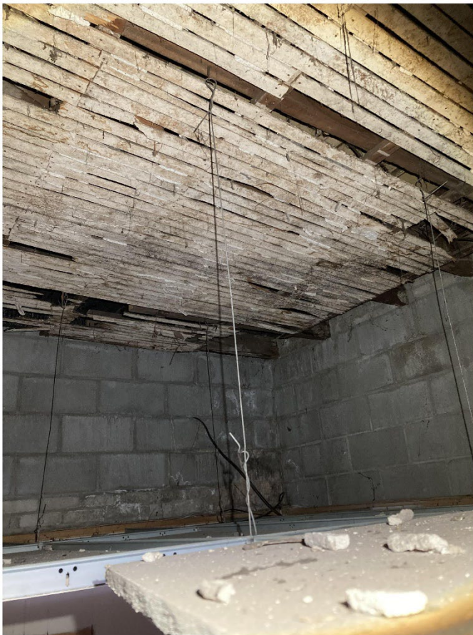
Photo 10 – Image taken above drop ceiling in Hope Barber Shop showing evidence of fire damage from the second floor portion being burned and the first floor surviving.
