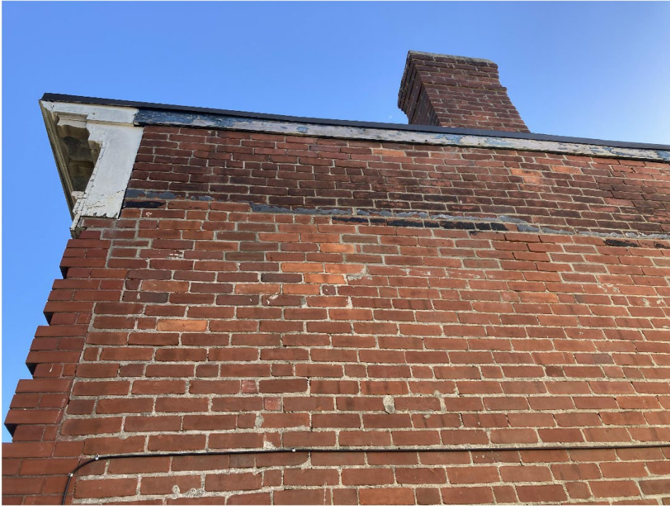
Photo 5 – Remnants on the brick showing location of non surviving roofline.
