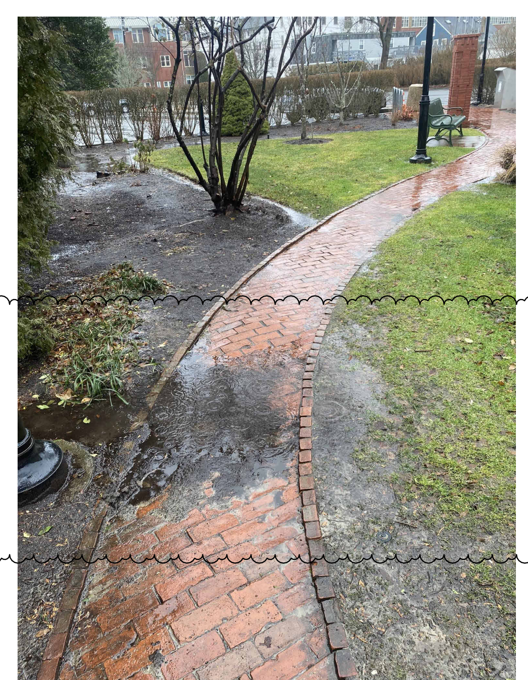
VIEW OF BRICK PATH AND PLANTING AREA AT SOUTHWEST CORNER OF THE PROPERTY. AREAS OF SETTLED BRICK ARE CAUSING WATER TO COLLECT ON THE BRICK PATH.
