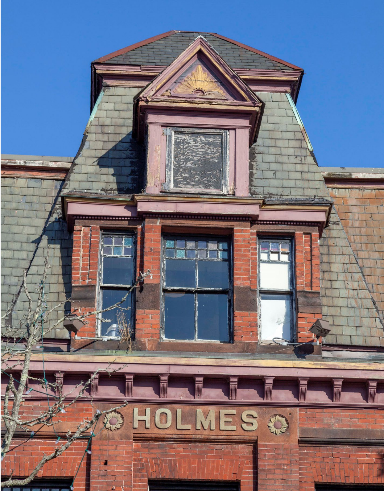
Photo 3 –Close up Image of Existing State Street Tower condition.
