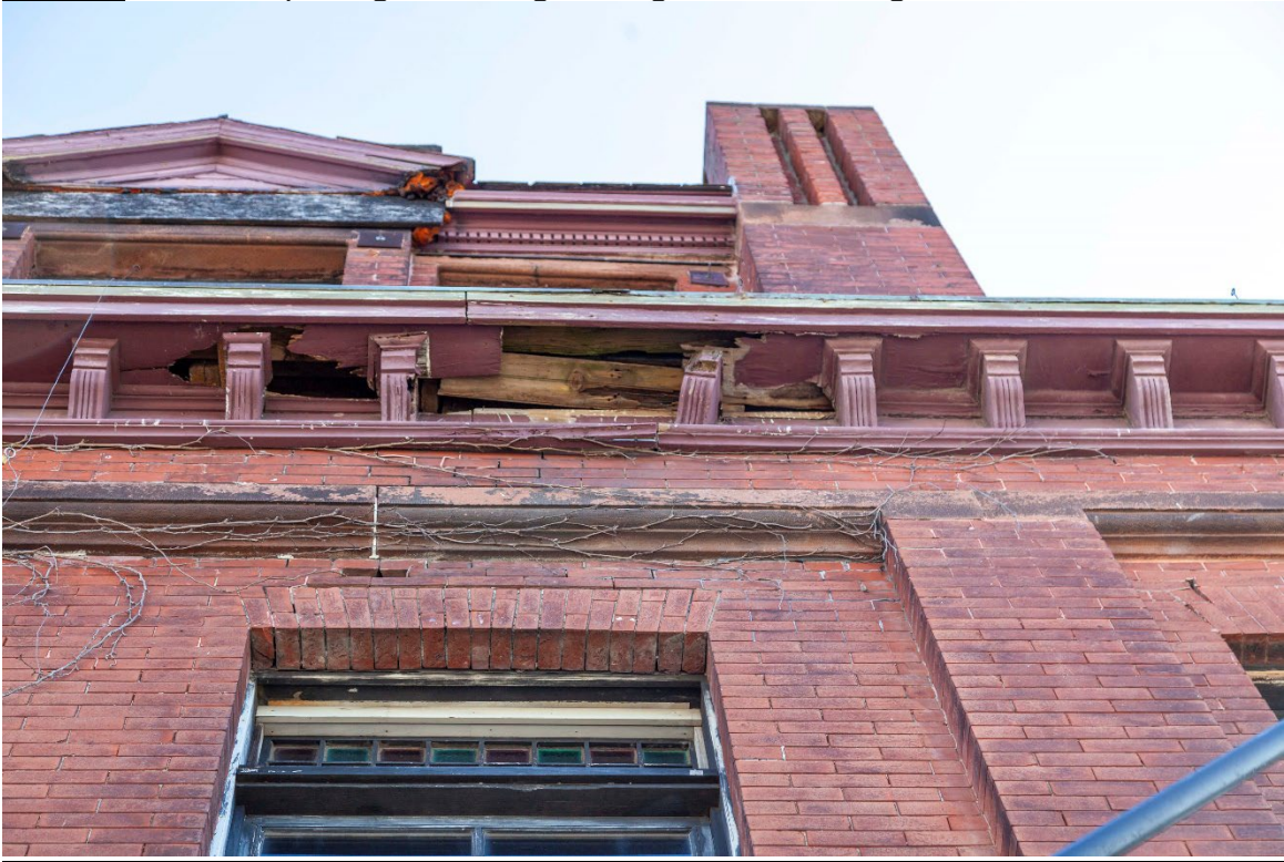
Photo 6 – Close up image showing damaged and missing wood elements.
