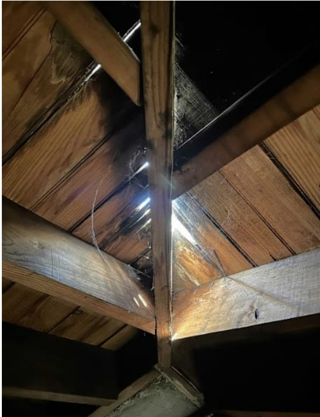
This photo shows deterioration of the house roof framing due to holes in the roof.
