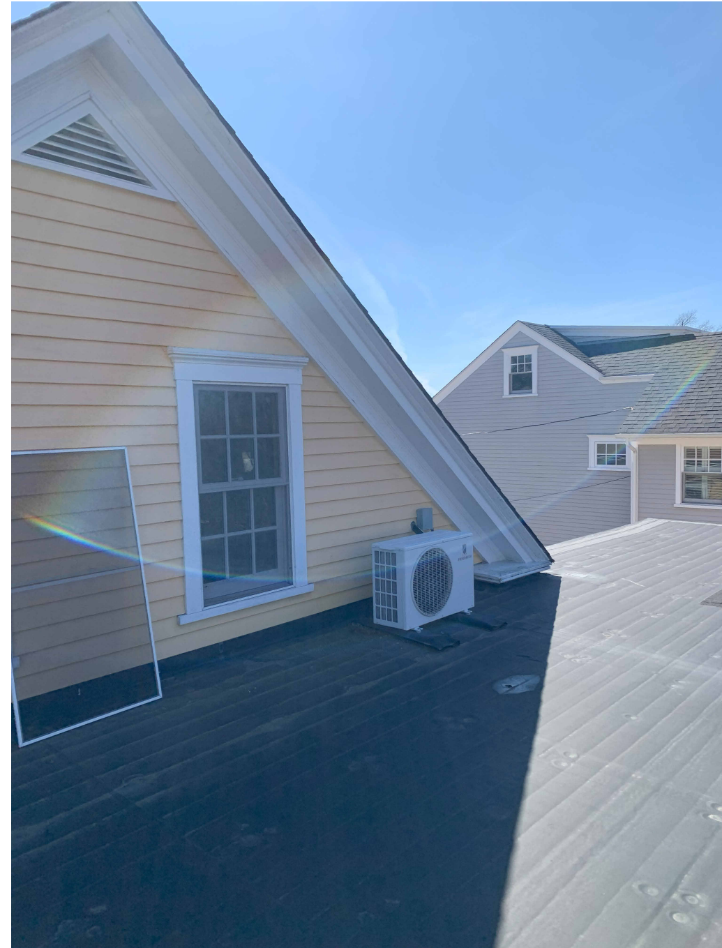
Photo #7: View of second floor condenser unit located on flat roof at rear of the home
