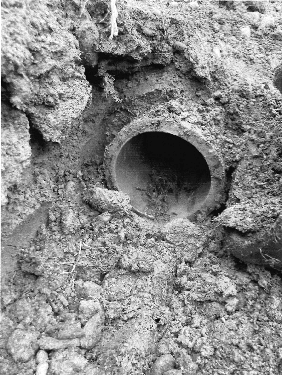
Root inside the pipe
