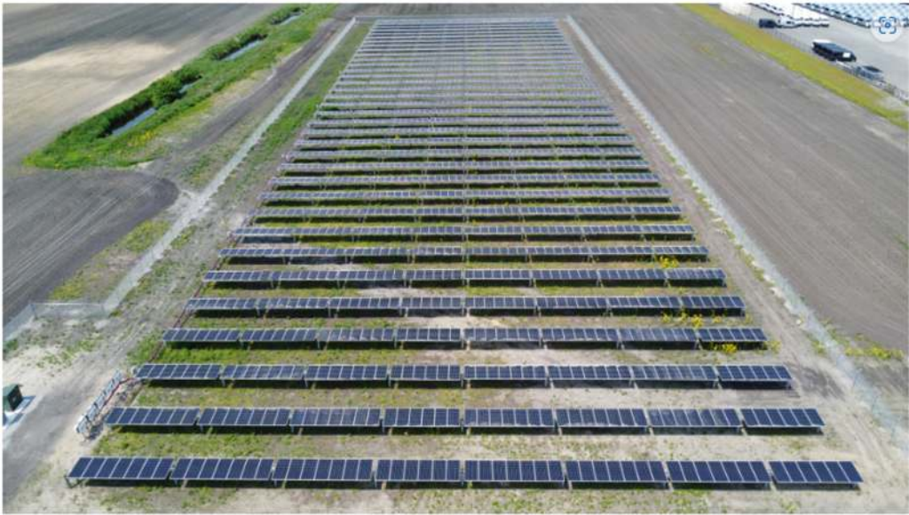
Valmont Industries, Inc., Solar Field
