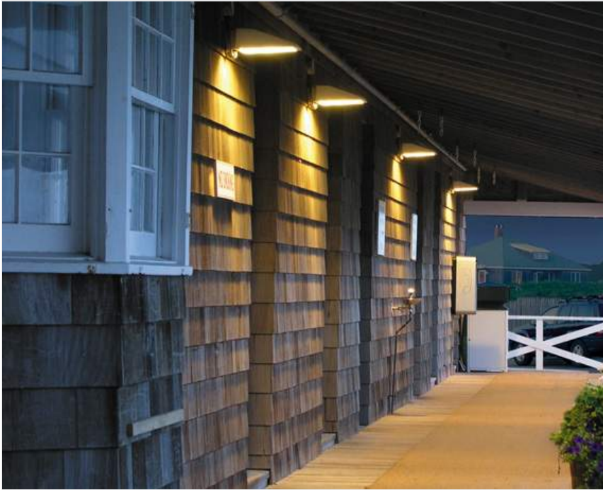
Commercial lighting should be Dark Sky compliant.
