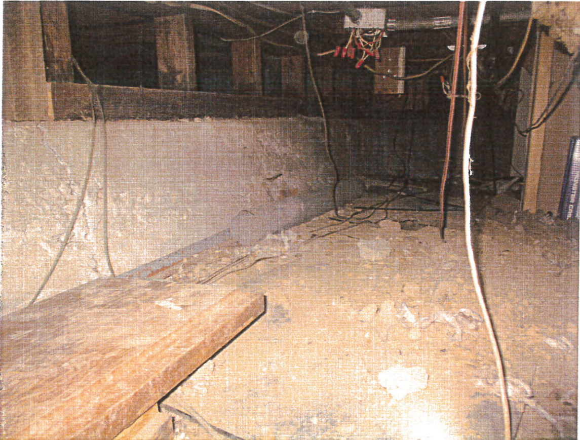
Photo 2: View within the foundation crawl space. Note the diagonal crack in the continuous interior footing near the left side of the photo.
