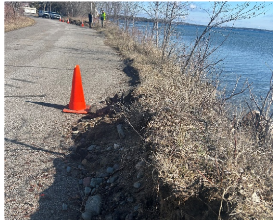
Figure 4: Shoreview Lane Damage – North Facing
