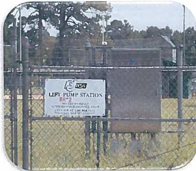
Figure 2- Pump Station that serves neighborhood
