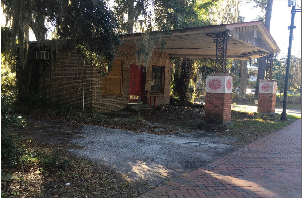
Figure 4.25 Constructed c. 1940 as a gas station (as evidenced by the porte cochere) within the Bluffton Historic District Survey Area (Resource 046-0105, Coburn Package Store, 1288 May River Road).
