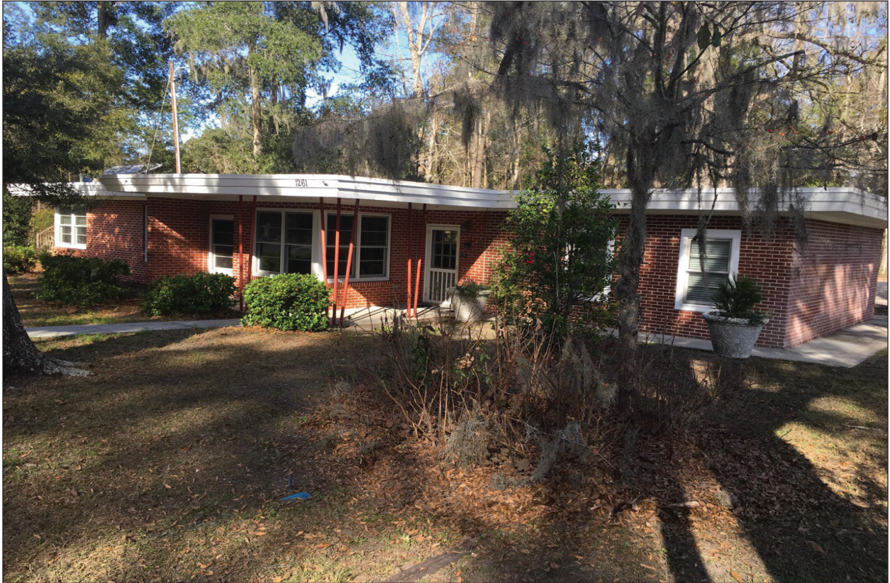
Figure 4.27 Resource 5287, 1261 May River Road, within the Bluffton Historic District Survey Area was originally constructed in 1957 as a clinic in a mid-century Modern style. This is evident in the flat roof, decorative metal roof supports, and corner windows.
