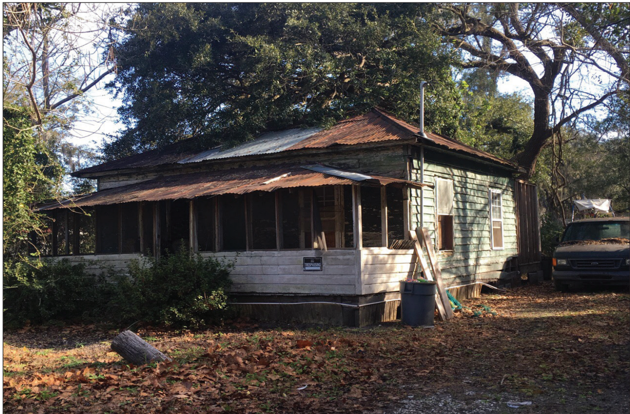
Figure 4.6 Example of a one-story pyramidal cottage within the Bluffton Historic District Survey Area (Resource 046-0096, the Frasier House, 3 Wharf Street).
