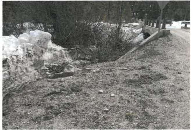
Figure 22. Damage to vegetation outside r-o-w and discharge of road base into Blue River. (May 5, 2024)
