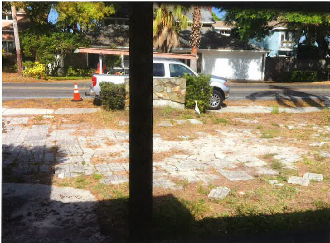
Photo 2: Broken and Loose Pavers, Overgrown and showing 5 ft wall.
