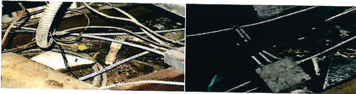
Lots of debris in the attic. Wiring is below the overflow pan. Potential electrical short if pan overflows. Insulation is torn off almost everywhere.
