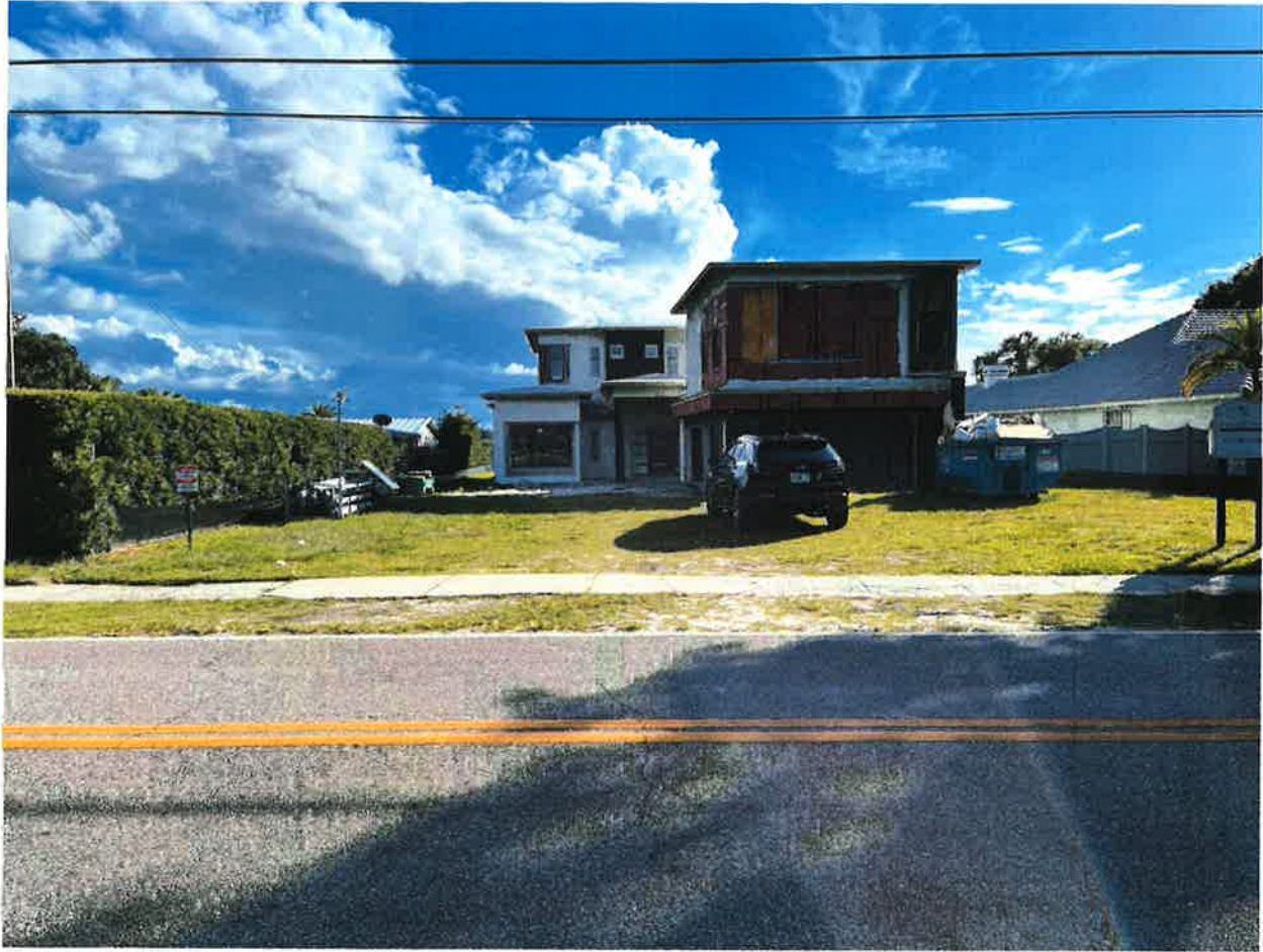
Subject Property 7208 Seminole Drive - 5' Black Aluminum Fence is already in front of the property from a previous permit
