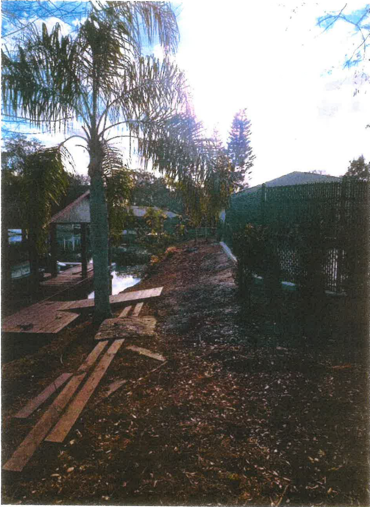
The grade of the access is very steep and will be steeper when backfilled and sod added
