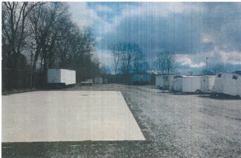
39'x97' Existing Concrete Slab. Looking from the west end of the property.
