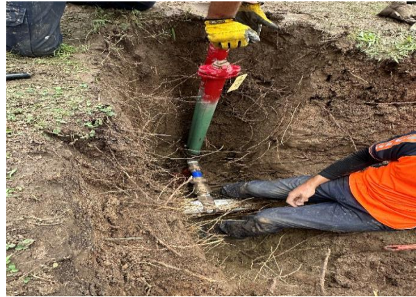
Flushing Hydrant Reck-
