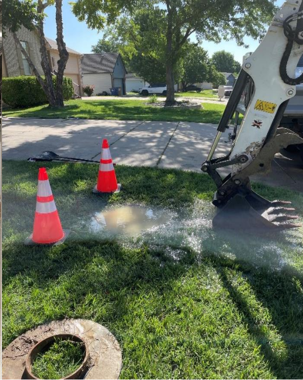
Water leak on main, St. James
