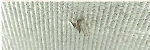
Roofing nails piercing roof decking
