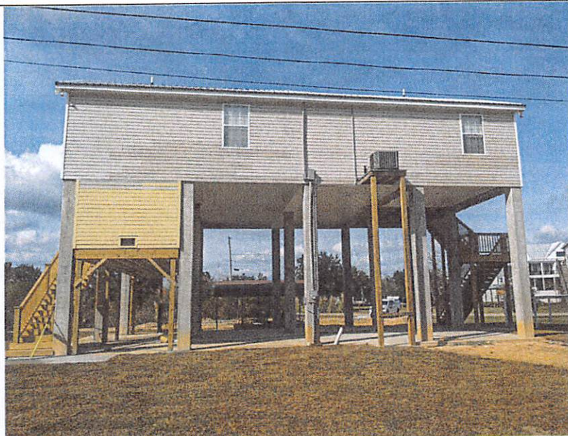
Photo Two Caption: South Side showing HVAC Equipment
