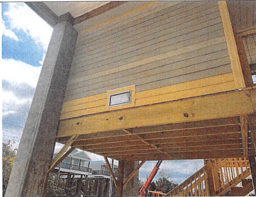
Photo Four Caption: Elevated Enclosure
