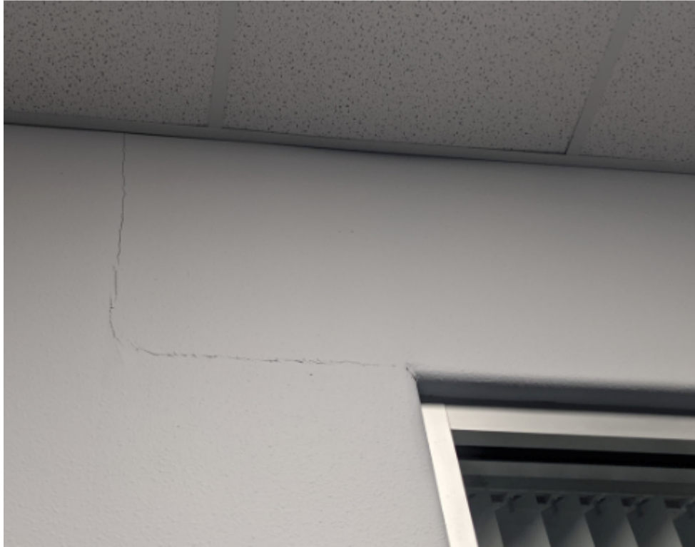
Figure 5 – Gypsum Wall Crack at Interior Wall
