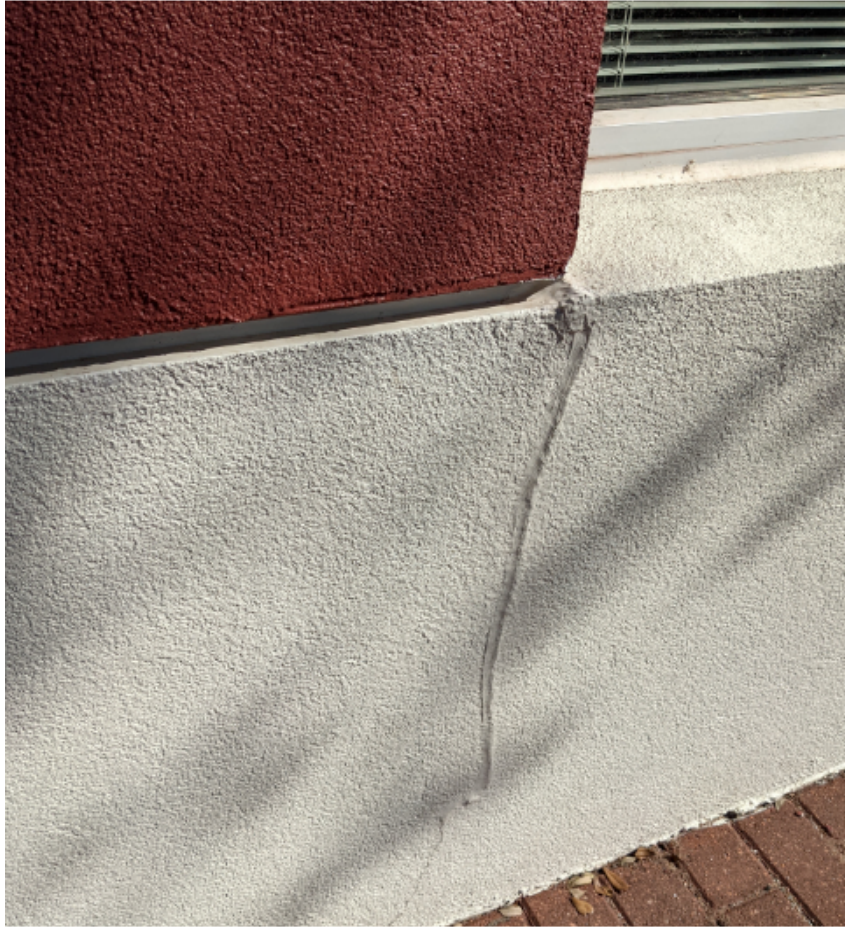
Figure 7 – Facade Crack at Exterior Wall (Near SE Corner of Building)
