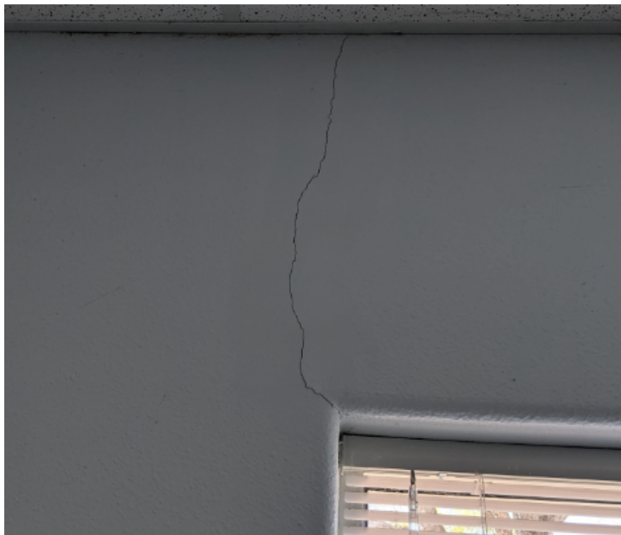
Figure 6 – Gypsum Wall Crack at Exterior Wall (Near SE Corner of Building)
