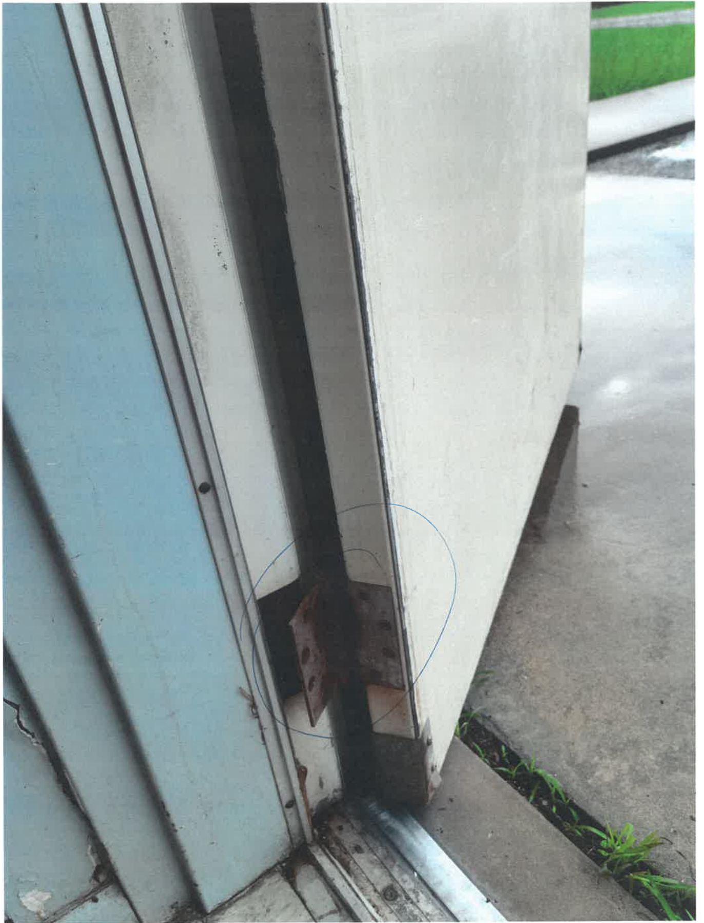
Rusted Hinges on Kitchen Entrance (All Hinges on exterior are rusted out)
