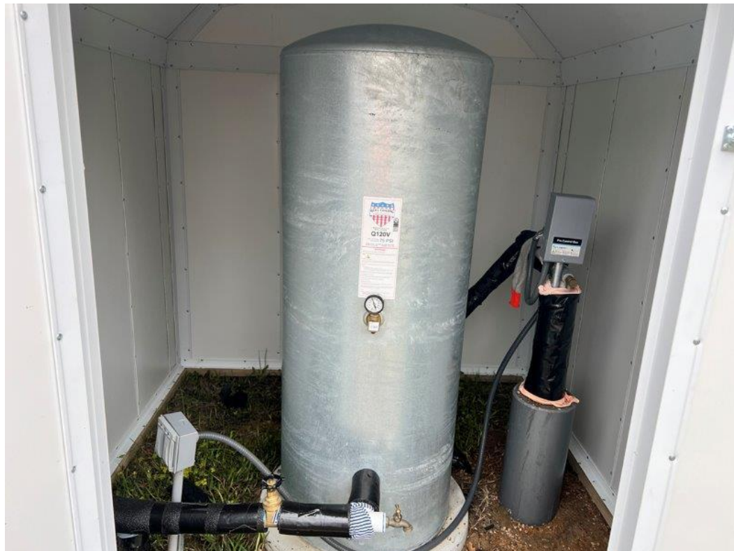
Photo No. 11: Well North pump / filter house
