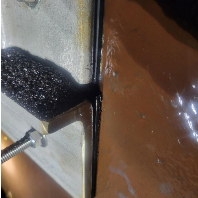
5. Gap in gasket at Filter 3.
