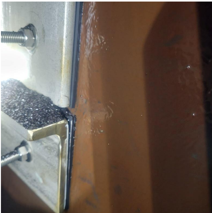
6. Gap in gasket at Filter 3.
