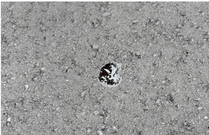
Photo 2 - Visible Mastic on Surface
