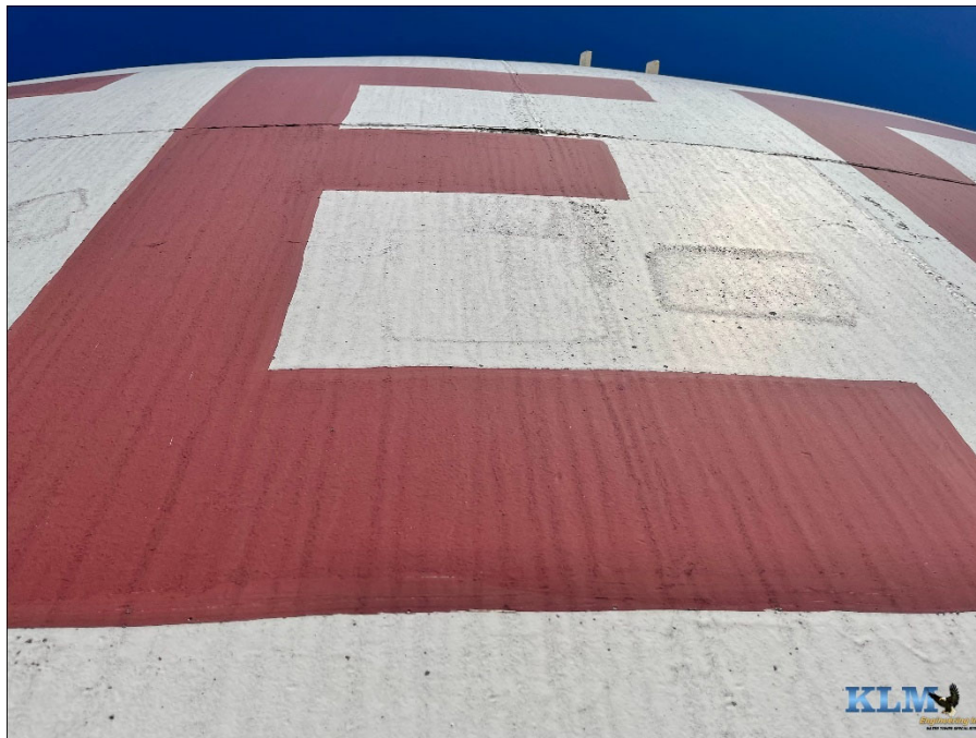
Photo No. 24 Shell coating conditions
