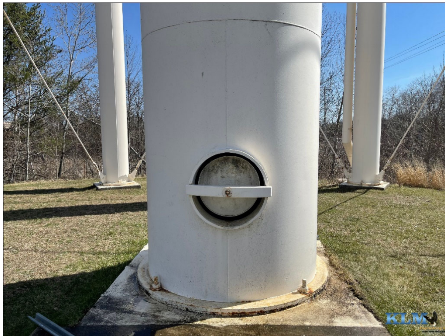
Photo No. 34 Base of wet riser
