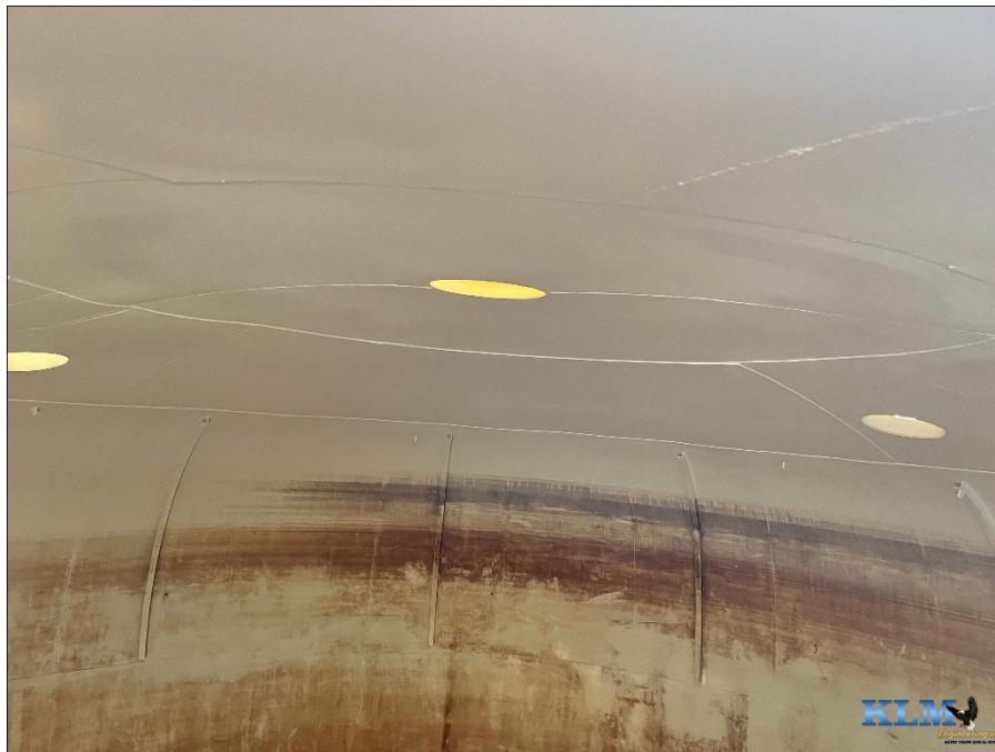
Photo No. 2 View of interior wet roof
