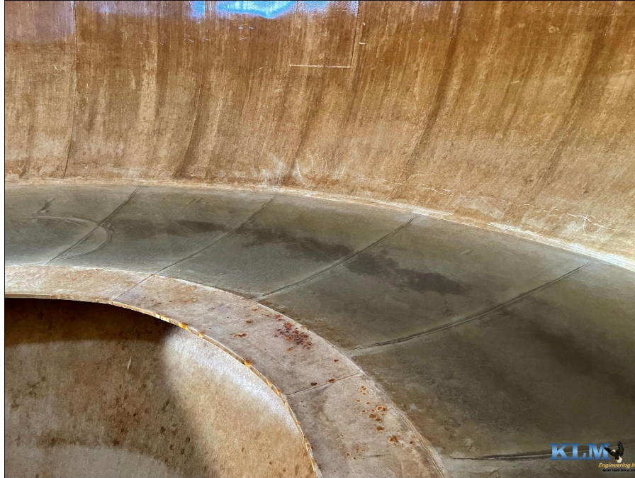
Photo No. 9 Bowl conditions Corrosion on bowl visible
