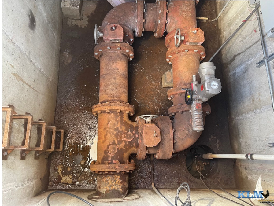
Photo No. 39 View of valve pit
