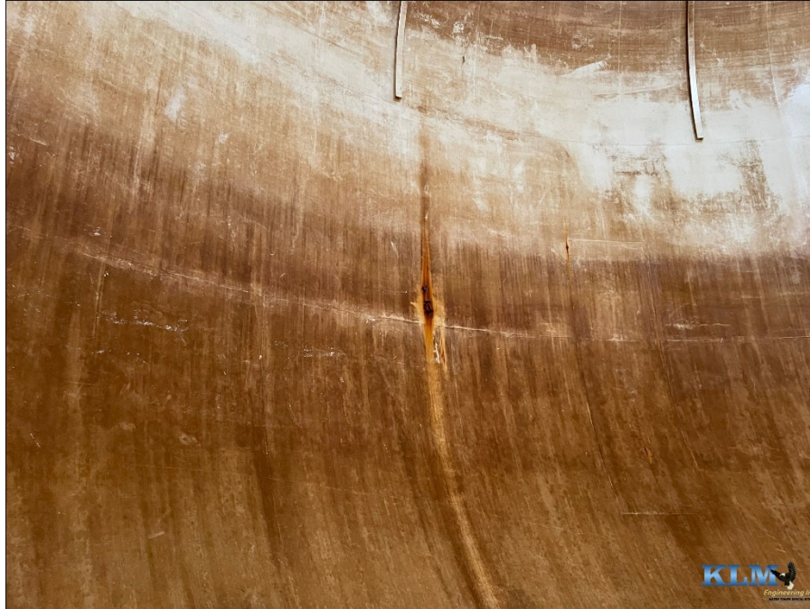
Photo No. 7 Shell coating conditions Large corrosion spot visible
