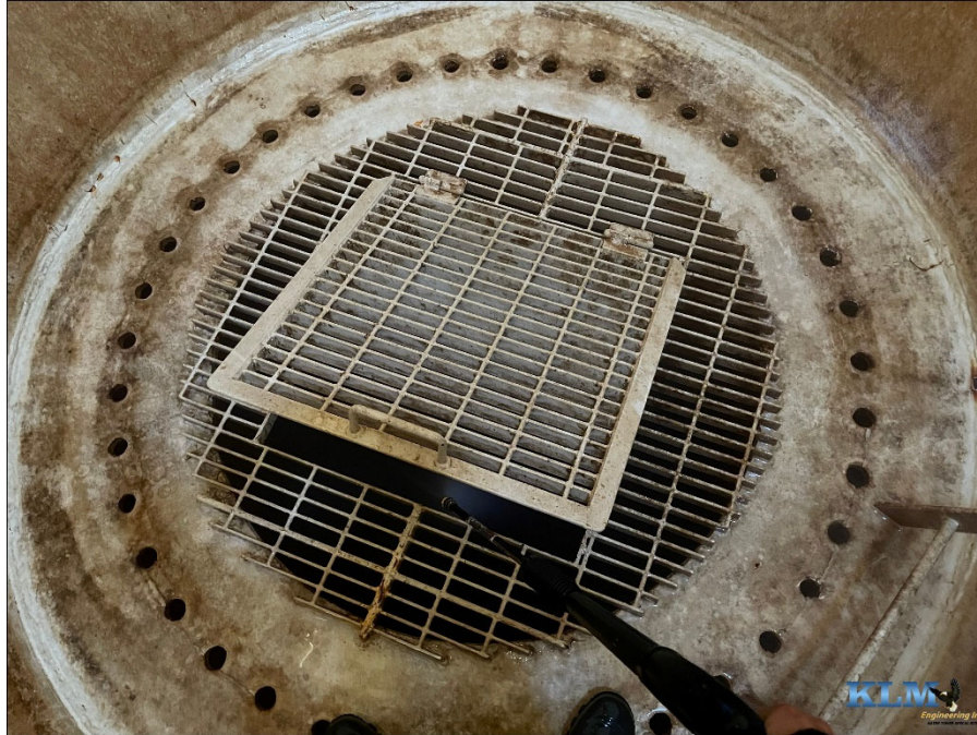
Photo No. 13 Condition of wet riser grating
