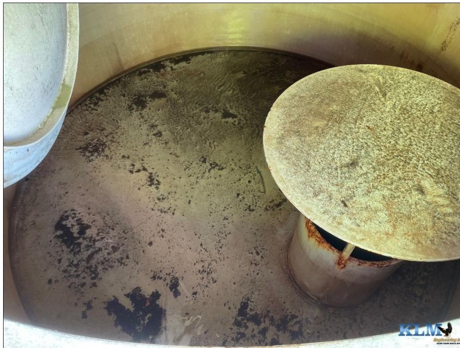
Photo No. 14 Bottom of wet riser
