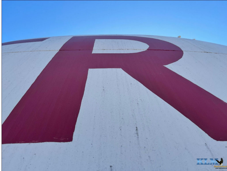
Photo No. 25 Shell coating conditions
