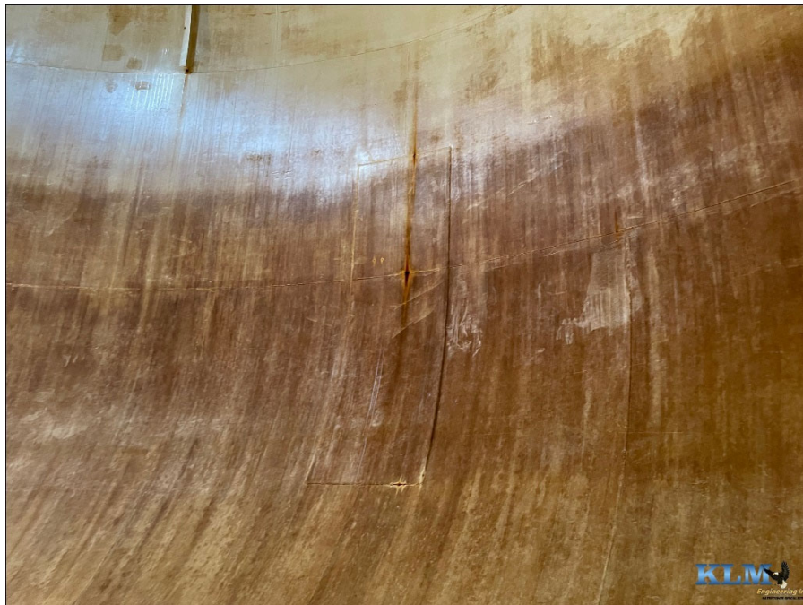
Photo No. 8 Shell coating conditions
