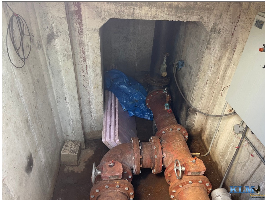
Photo No. 40 View of valve pit
