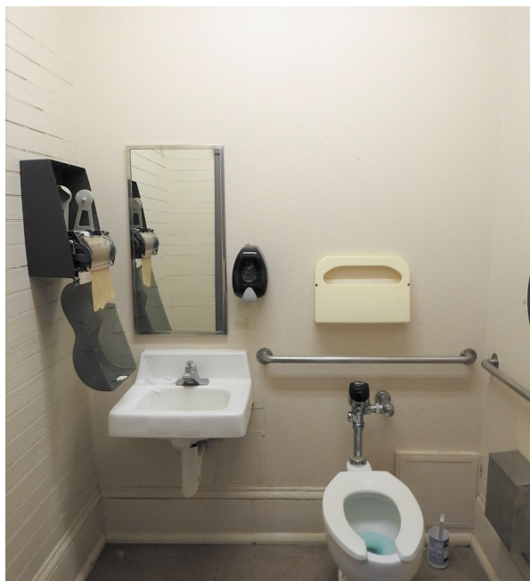
Photo 13: Existing non-ADA compliant 1 st floor restroom.
