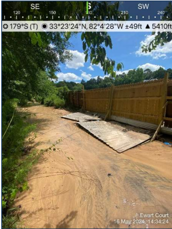
Photograph 1: 2010 Ewart Court, looking upstream at the left bank adjacent to the failing fence line.
